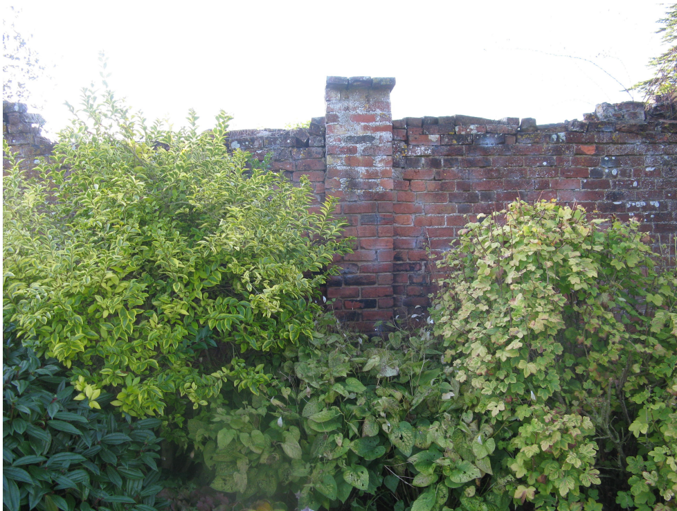
Plate 3 - Column (Q) with damaged wall looking south
