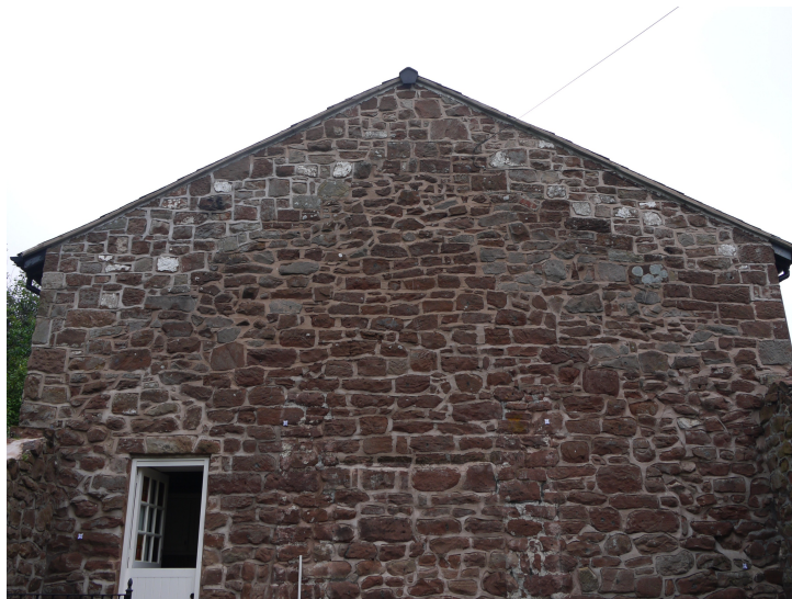
Plate 2 - Roof scar on southwestern elevation
