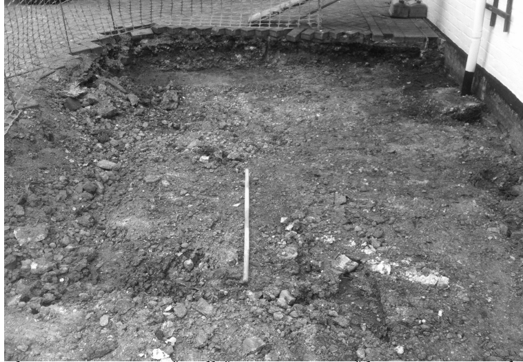
Plate 1: Excavation of wall footing at west of house. Facing north, 1m scale
