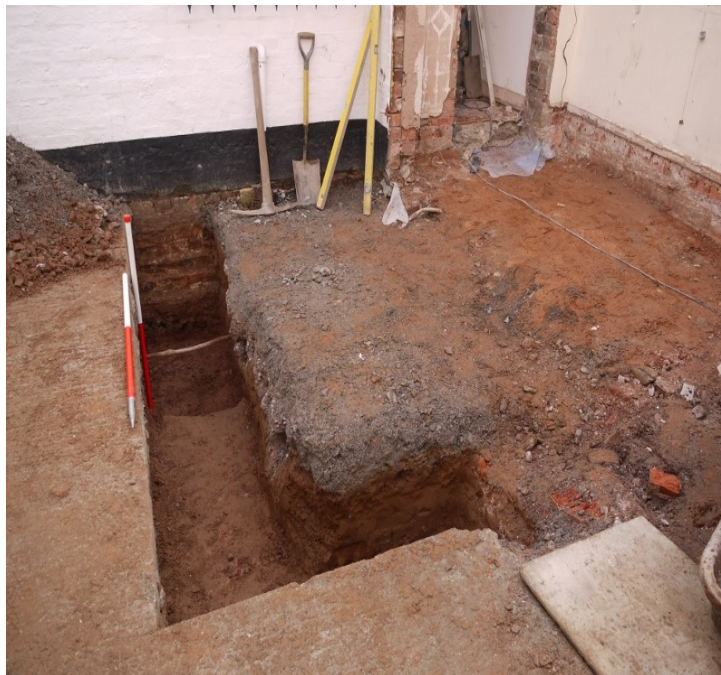
Plate 1 - View of the new foundation trench at the rear of 'the Bungalow' Looking south-east.
