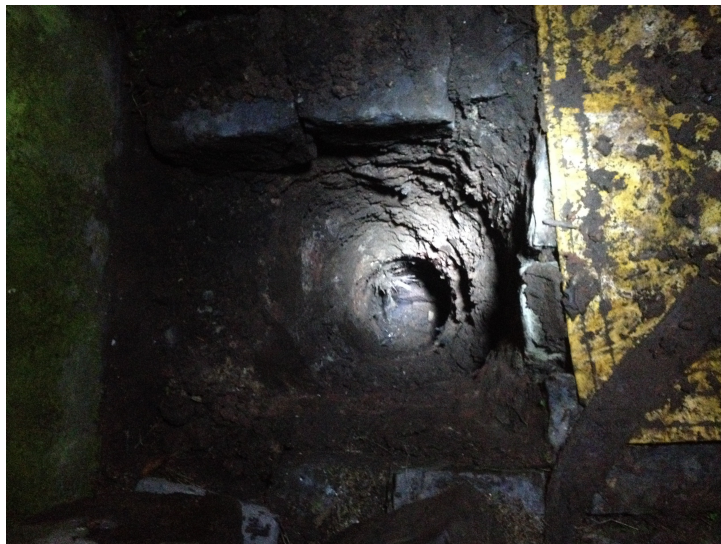
Plate 2 - Void created by removal of pole
