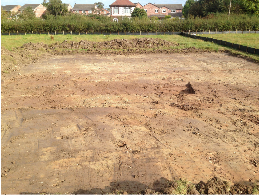
Plate 1: View of the area after topsoil stripping; Looking east. The field ditch is visible running across the centre of the area from left to right.
