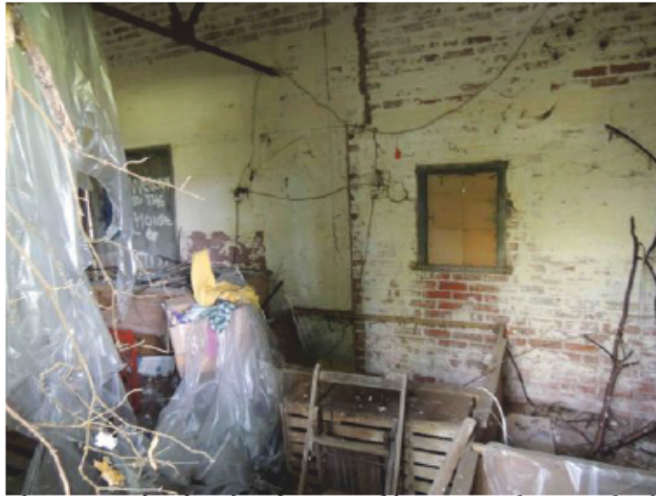
Plate 47 - Abandoned Military Building Internal, Osea Island
