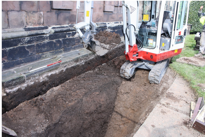
Plate 1 - Shot of trench excavation, showing southeast facing section of narrow excavation, looking north with 1m scale
