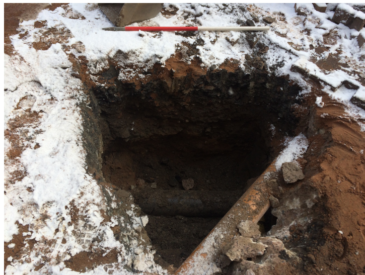
Plate 5 - Excavation of Trench 6 showing plastic drain pipe and gas service at the base.
