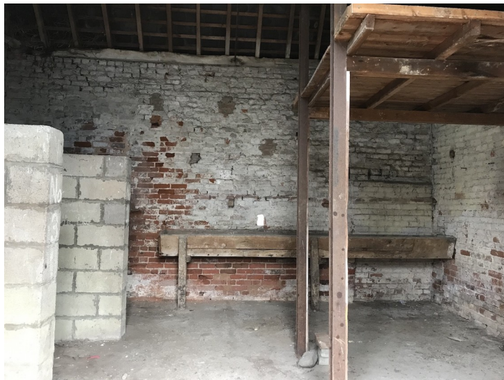
Plate 33- Building E, room 4 with breeze block stalls and animal feeder. Facing north.
