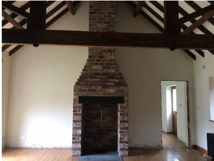
Plate 19- Building D, central open area with inserted chimney. Facing north, 1m scale.
