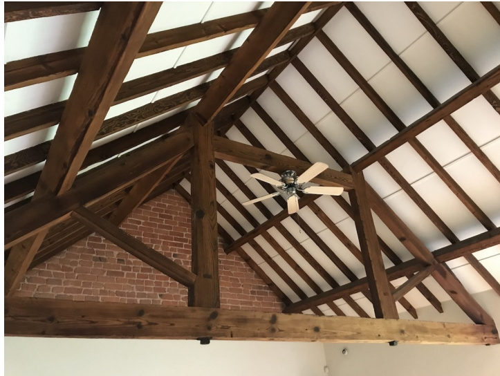
Plate 21- Building D, timber roof beam in the central open area. Facing southwest.
