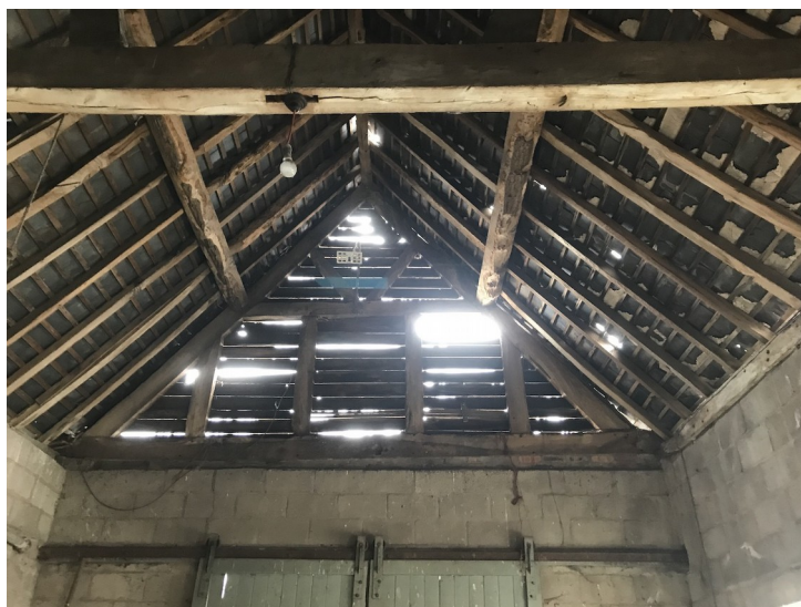
Plate 26- Building E, room 1 the internal facade of the east elevation. Facing east.
