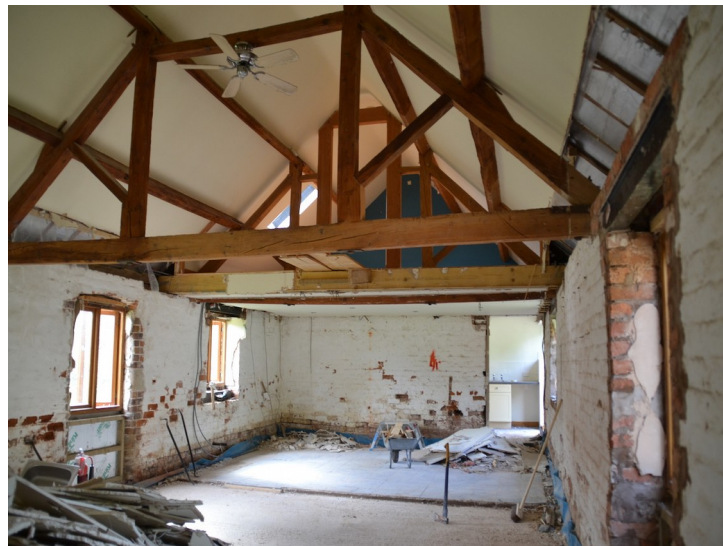
Plate 6- Building B, internal southern area, looking south to mezzanine area and doorway to extension.
