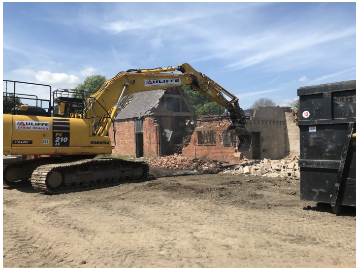
Plate 35- Building E, multiple phases and materials of construction seen during demolition. Facing northwest.
