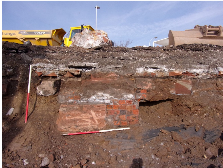
Plate 11- Sandstone and Brick footing [515] north of dock wall [504]. Looking north, 1m scale.
