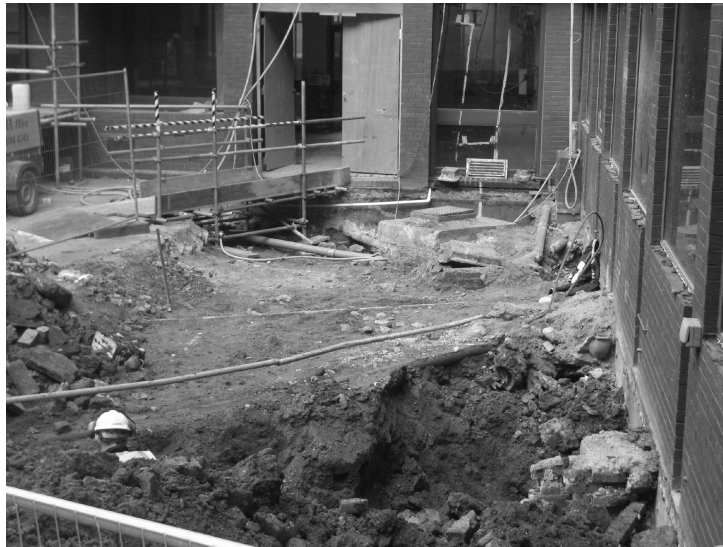
Plate 4 - South of the site area facing north, showing the extensive services in the area and the depth of truncation in the trench in the foreground.
