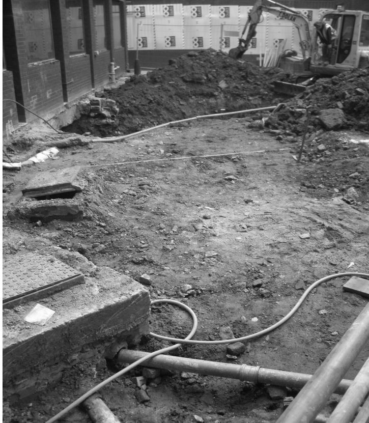
Plate 1 - North of the site area facing south, showing the extensive services in the area.
