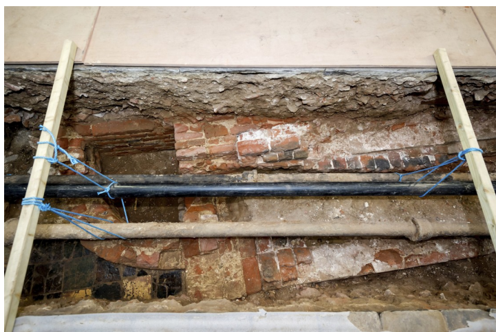
Plate 8 - The north side of the chimney breast {SGR: 54}, with the internal hearth structure {SGR: 55} to the south of it. To the north glazed tile floor {SGR: 61} and structure {SGR: 60} area also visible. Photograph taken facing east, no scale.
