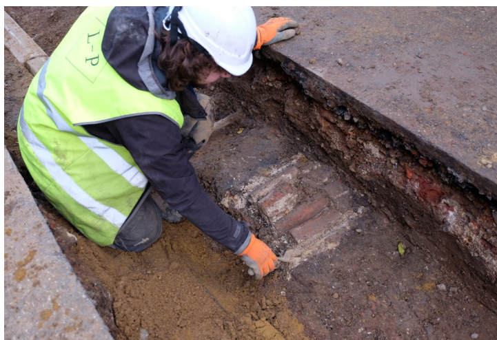
Plate 3 - The excavation of culvert {SGR: 16}, the culvert had been truncated to the south by the cut for an electrical cable. Photograph facing north-west, working shot featuring Aaron Clarke.
