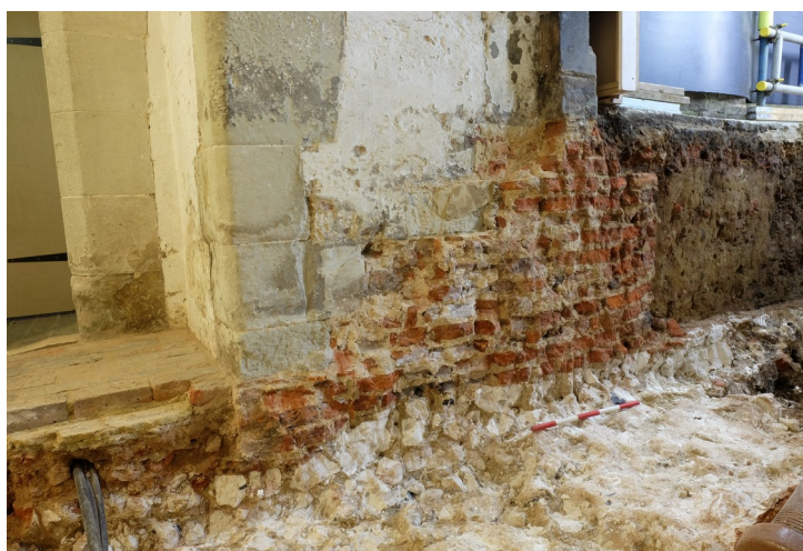
Plate 17 - Foundations for the Henrician Great Hall {SGR: 70}, seen in section following the removal of the stairs Photograph taken facing north-west, 0.5m scale.
