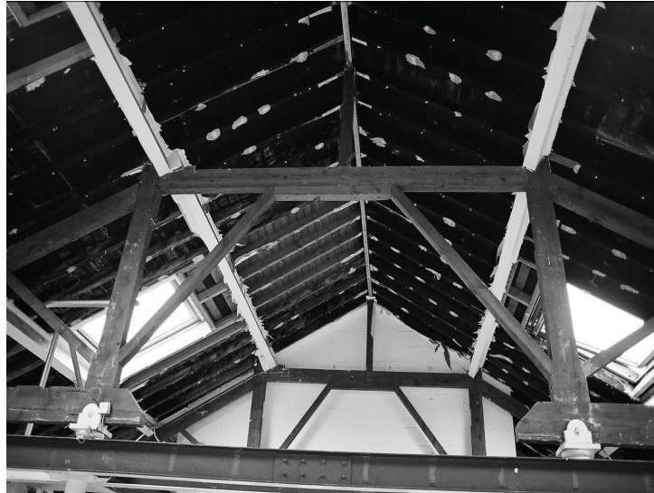
Plate 18 - Roof truss in 3.1. Note modern addition of steel joist, and original open tie-beam arrangement.
