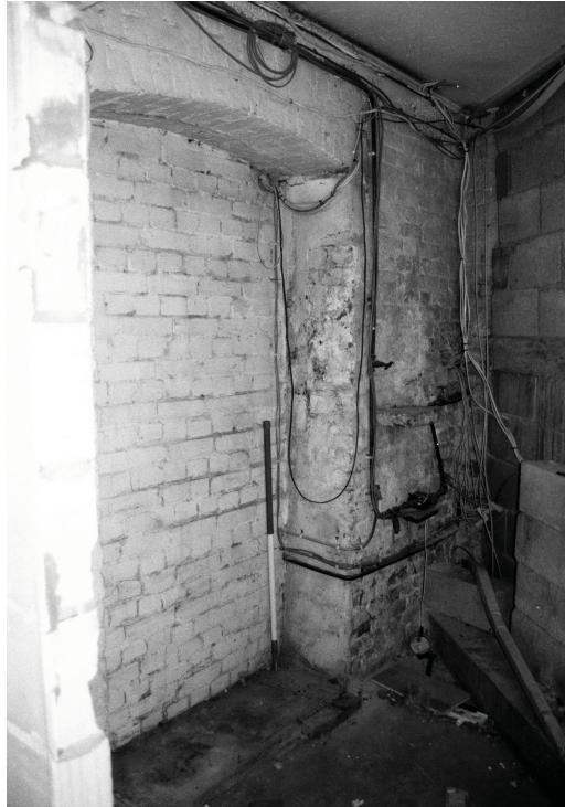
Plate 7 - View of the blocked doorway in B.6, viewed from the doorway to B.7. On the right, the diagonal breezeblock wall described in the text.
