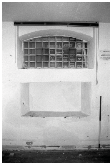
Plate 5 - Detail of the window recess in bay 6 of the east wall in room B.3.
