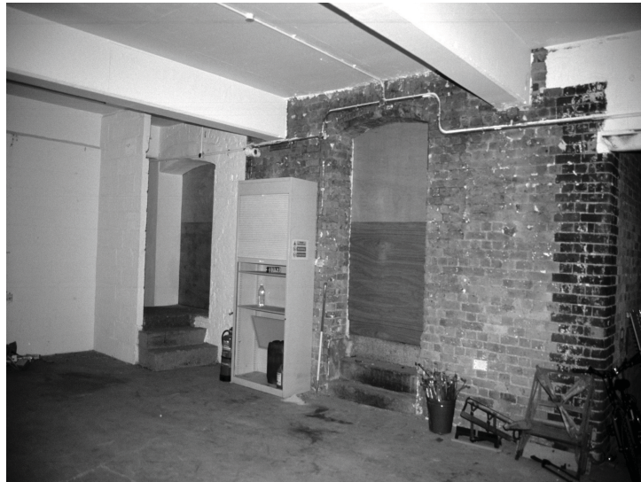
Plate 13 - View of the south west corner of the historic core building, seen from G.7. Note the two modified window apertures, bay 2 foreground bay 3 in distance .
