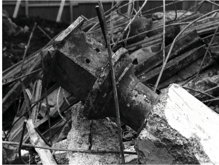
Plate 23 - Cast iron column after demolition. Concrete casing has broken away from the capital, but remains in place on the shaft.
