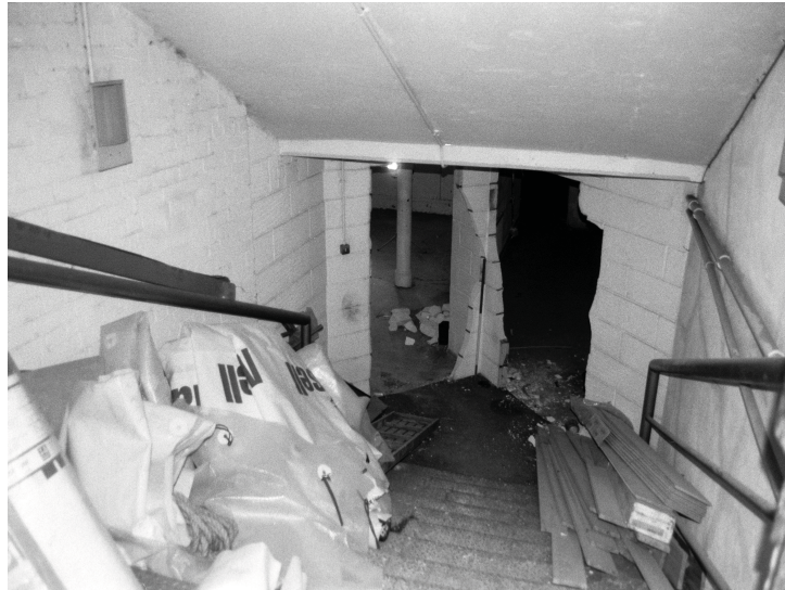
Plate 3 - The view down from pavement level to basement level in space B.1.
