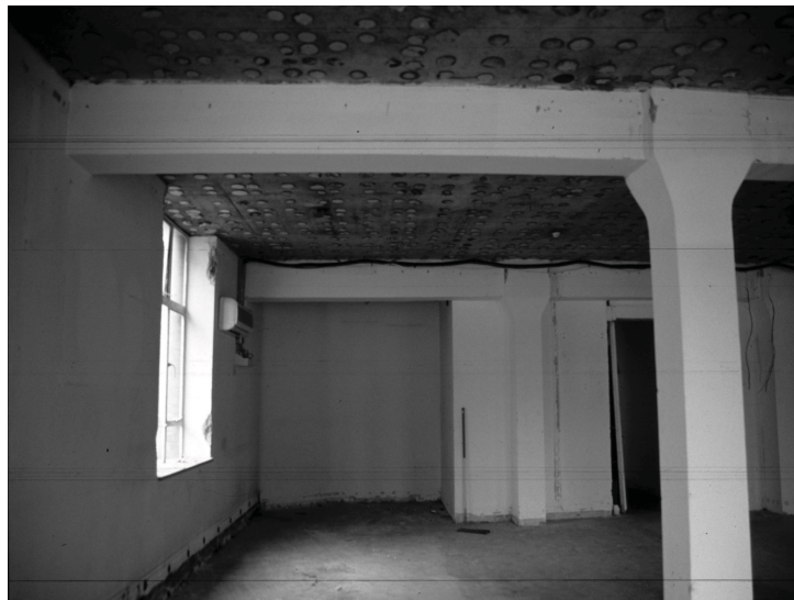
Plate 17 - View of 2.1 looking south along the east bay. Note window (east facade) and columns.
