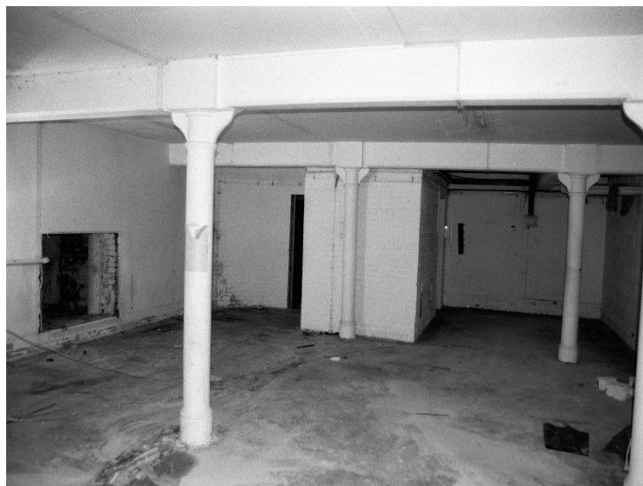
Plate 4 - View from the north west corner of B.3 looking across bays 6 and 5 towards the lift block in bay 4. Note also the recess in bay 5 of the east wall (left).
