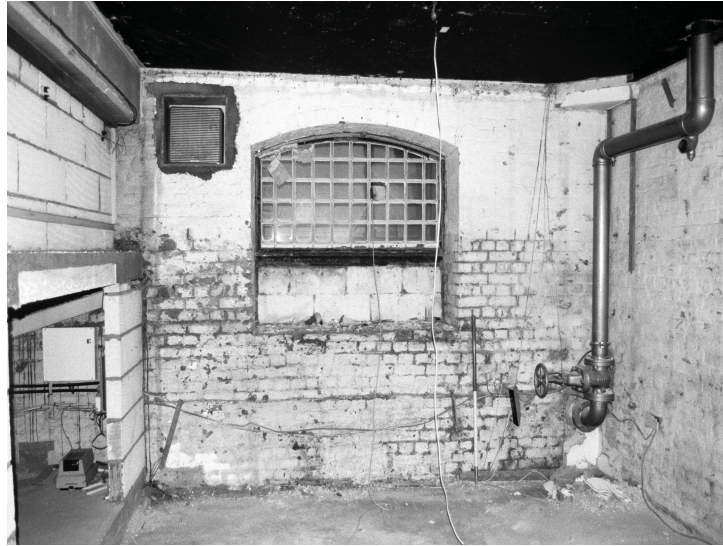
Plate 8 - The east wall of B.8. Showing the window detail, as well as the undercroft area (on left). Ventilator (top left of window). Sprinkler system valve (on right) and the base of the G.5 fireplace (top right corner of the room).
