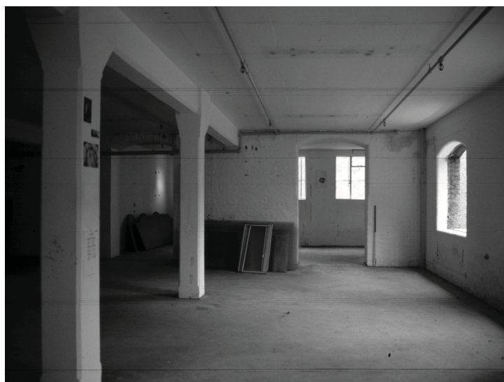
Plate 14 - Room 1.1, bay 6 looking west towards room 1.2. Note modified window aperture and columns.
