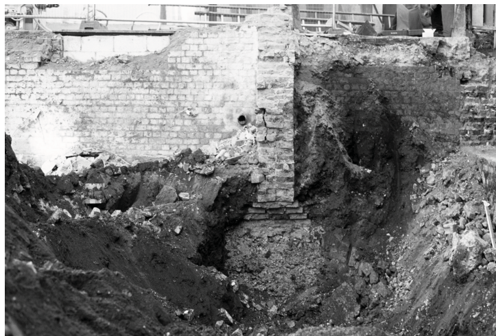
Plate 24 - Area bay 1 and 2 looking east. Wall with underpinning.
