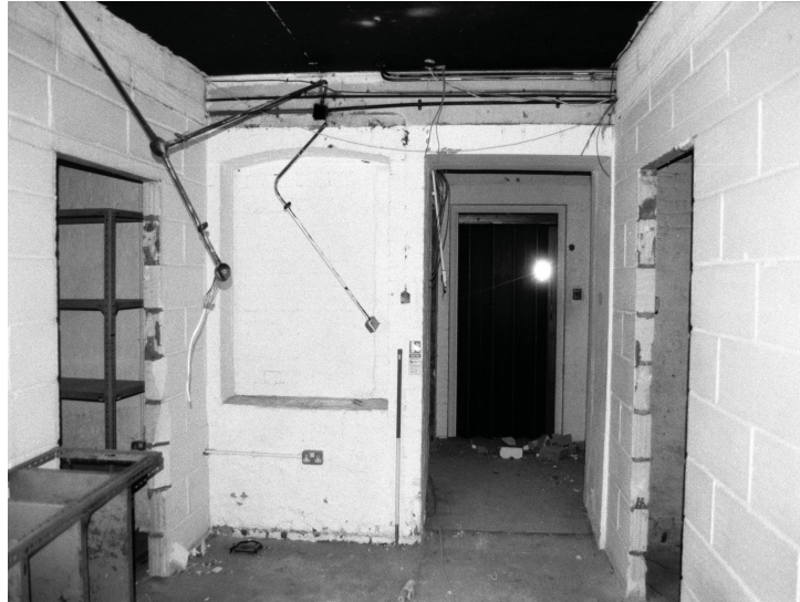
Plate 6 - View north from the doorway of B.8-B.7 towards B.4. Note the lift in the distance as well as the blocked window to the left of the doorway. The doorway on the left leads to B.9 and the doorway on the right leads to B.6.
