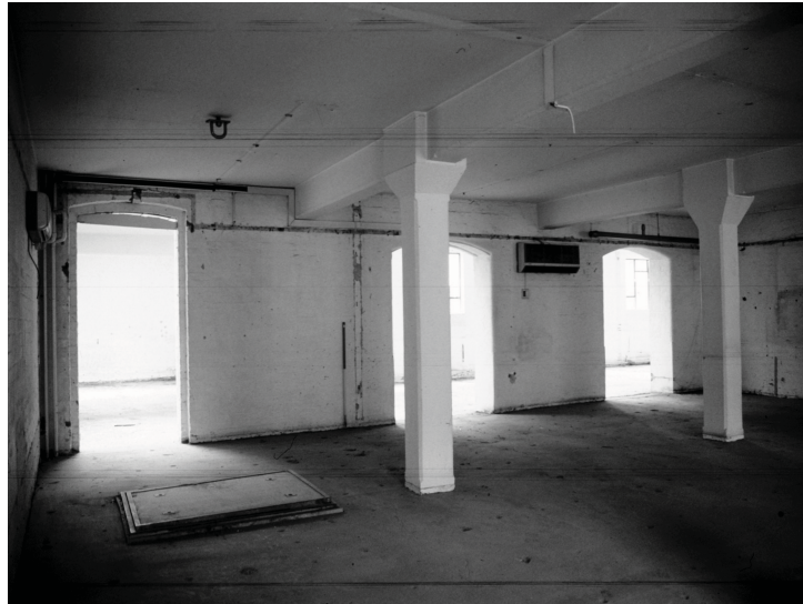
Plate 15 - View of 1.3 from the south east corner, looking towards 1.4. Note atypical doorway in bay 1 (left)
