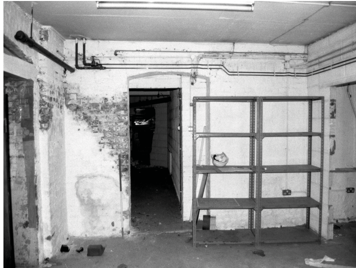
Plate 10 - South wall of B.9, this is the spine wall. Note the partially blocked original aperture. Also on far left of frame, a recessed area.
