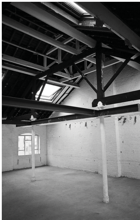
Plate 19 - Bay 1 in room 3.2. Shows window, truss, mezzanine floor joists and brick pier in south wall.
