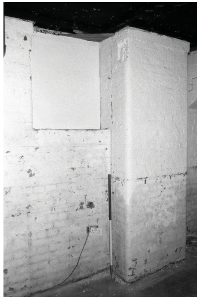
Plate 9 - Blocked window, brick pier and at extreme right, the base of a staircase. All features located in the south wall of B.8.
