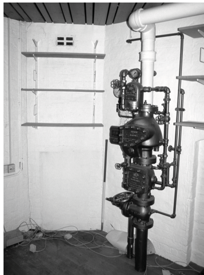
Plate 12 - Sprinkler equipment and blocked fireplace in G.5
