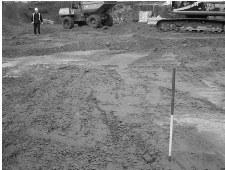
Plate 2 - The southern area of the study site, with context (108) being graded down to reveal the natural gravels and sands. 1m scale, north facing.
