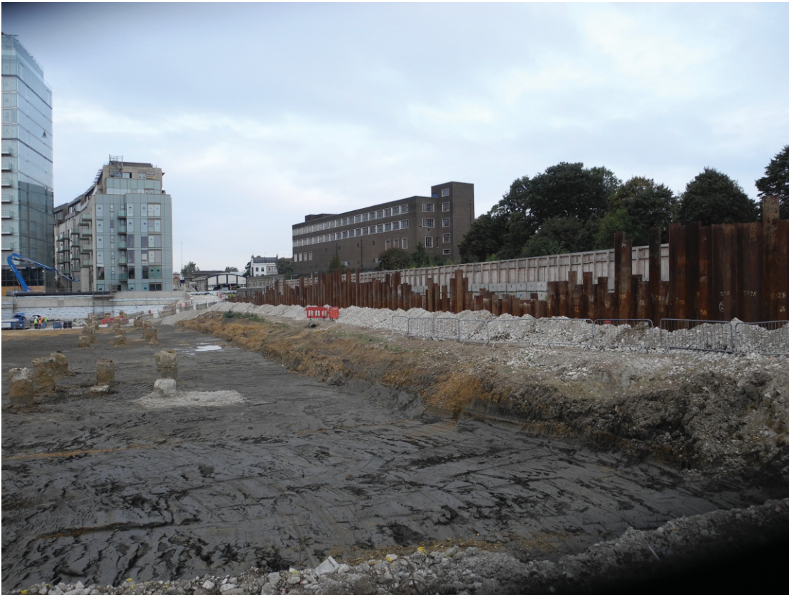
Fig 4 London Clay exposed below natural gravels at the east of the Phase 2 area, looking north
