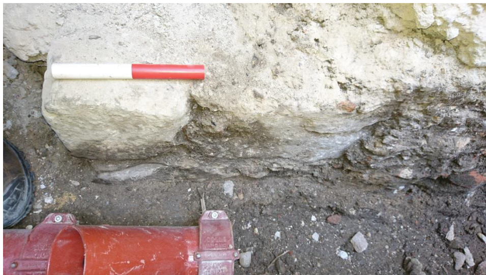
Fig 7 Detail of ashlar foundation at north-west corner of St Mary Somerset (0.2m scale)
