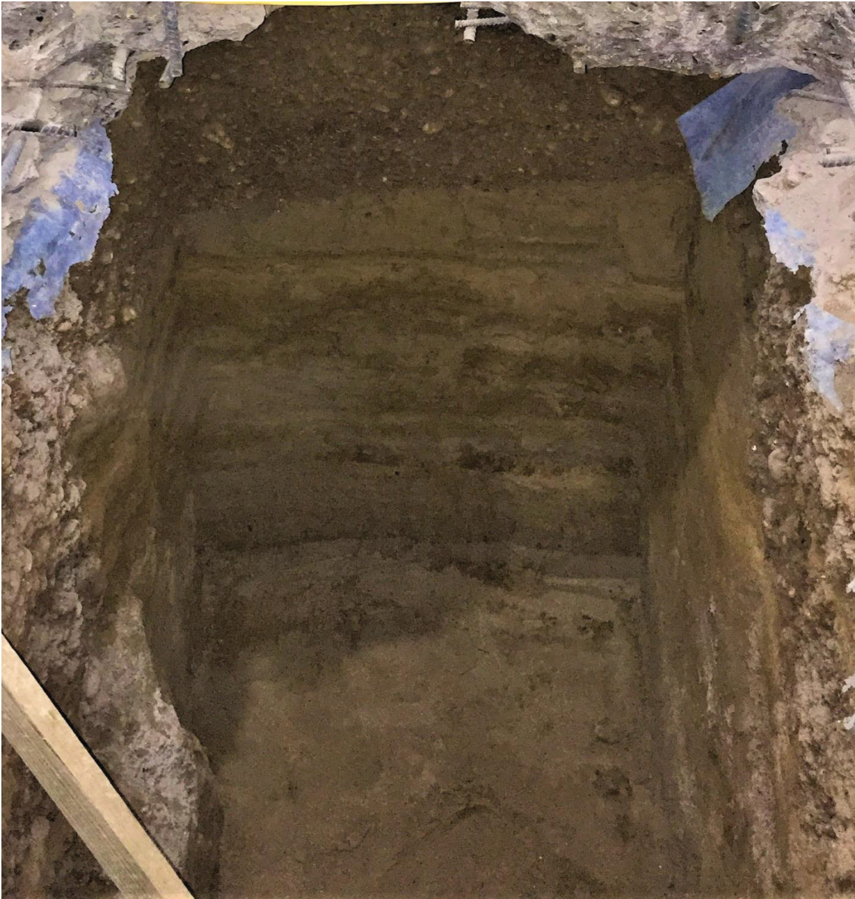
Photo 2 U-pin hole, looking west
