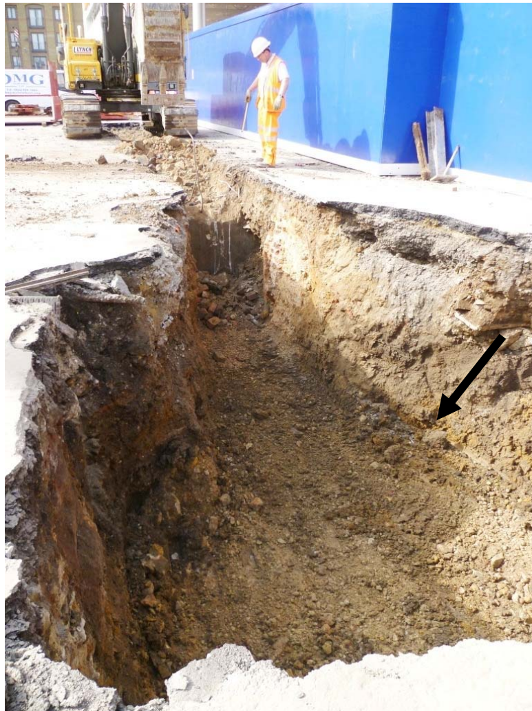
Photo 6: Eastern Manhole and Drainage trench: Looking west, showing Albion Brewery brick and concrete foundations cutting through archaeologically sterile natural deposits with a blackish waterlain silt (arrowed), cut through by Albion Brewery basements in the distance
