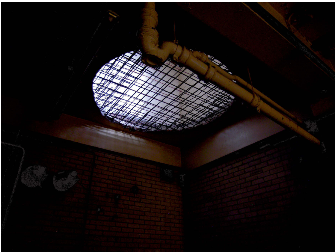
Fig 27 The circular hole cut into the concrete slab between the 5th and 6th floors of Area 3, looking north west
