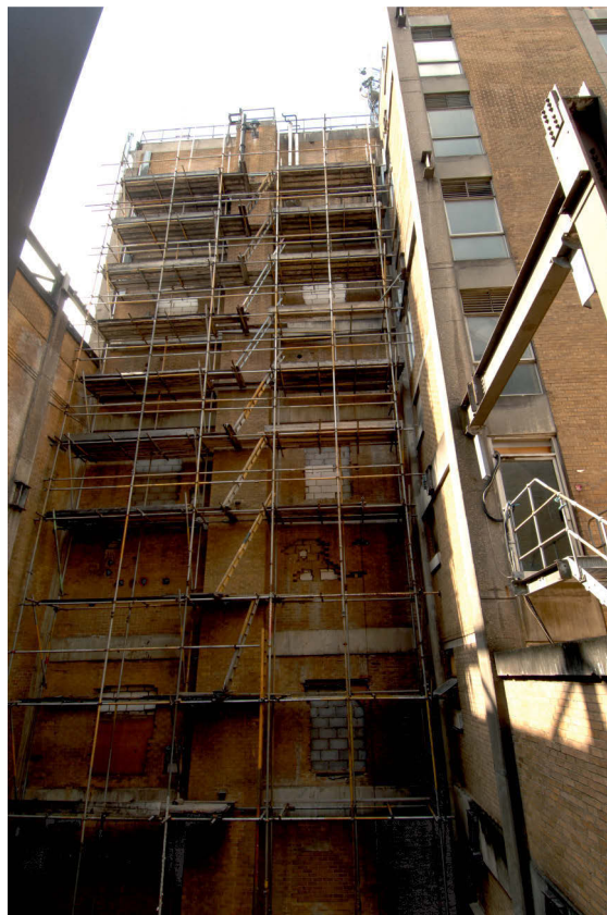
Fig 31 The north wall of the easternmost part of Area 3, looking south over Open Area 5. Note the RSJs on the right of the photo
