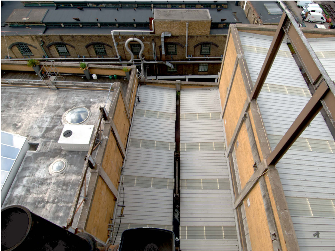
Fig 16 The roof of Area 2, viewed looking south from the roof of Area 3
