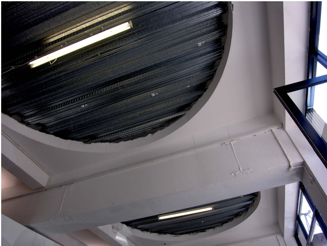
Fig 11 The ground floor ceiling of Area 1, showing the circular holes for the vats & the cut end of an RSJ, looking south
