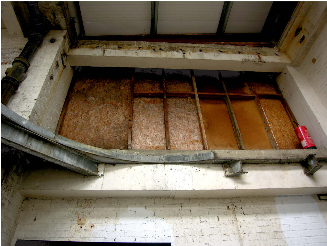
Fig 19 The former 3rd-floor access from Area 1 into the vat area of Area 2
