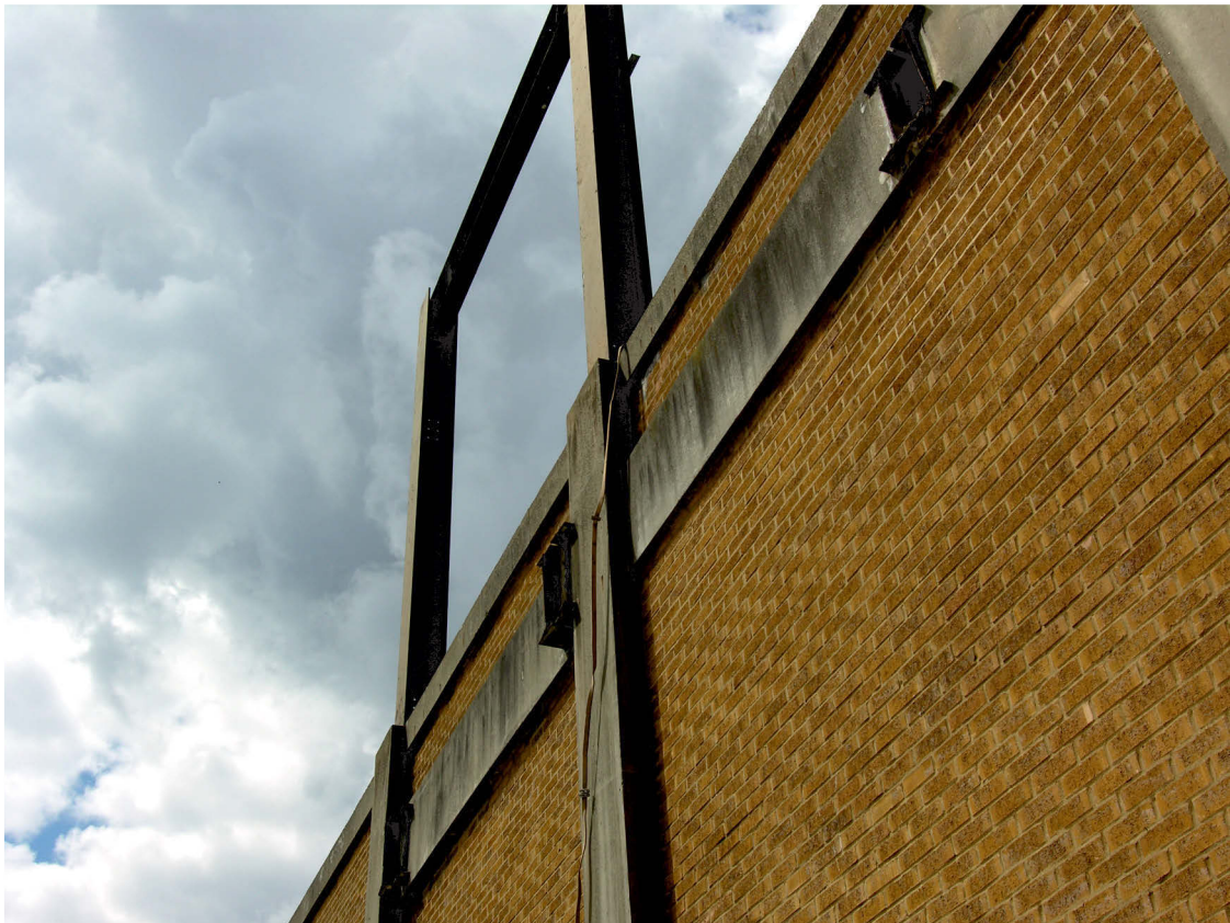
Fig 17 Steel columns and the cut ends of steel joists, emanating from the east wall of Area 1 looking south west, traces of a former structure in the space over Area 2
