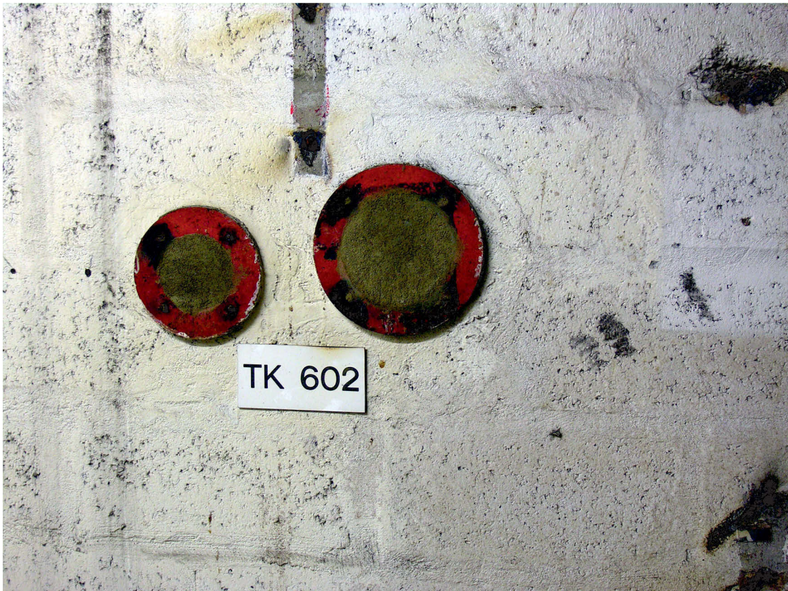
Fig 29 A blocked hole for a former pipe, labelled with a tank number, south wall of the 5th floor, Area 3
