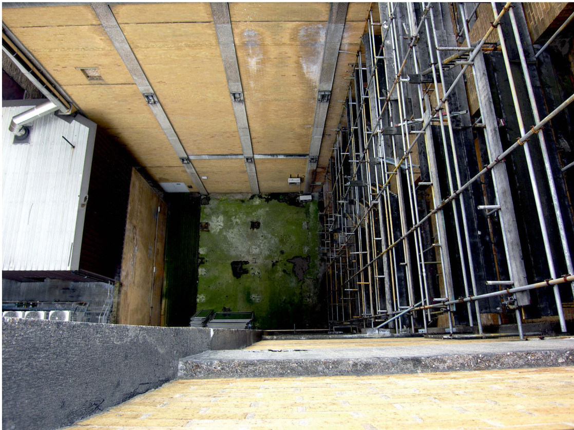
Fig 33 The view down into Area 5 from the roof of area 3. Note the cut ends of RSJs within the west wall of the adjacent Block D
