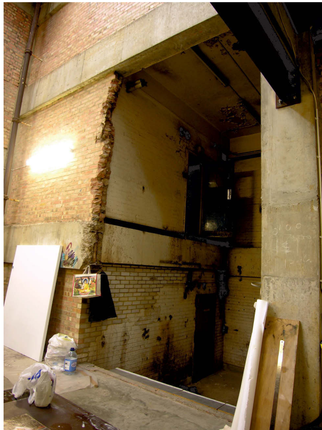
Fig 13 The view north from Area 1 into Area 3, through a recent opening in the wall, showing the difference in floor levels and the removed floor in Area 3
