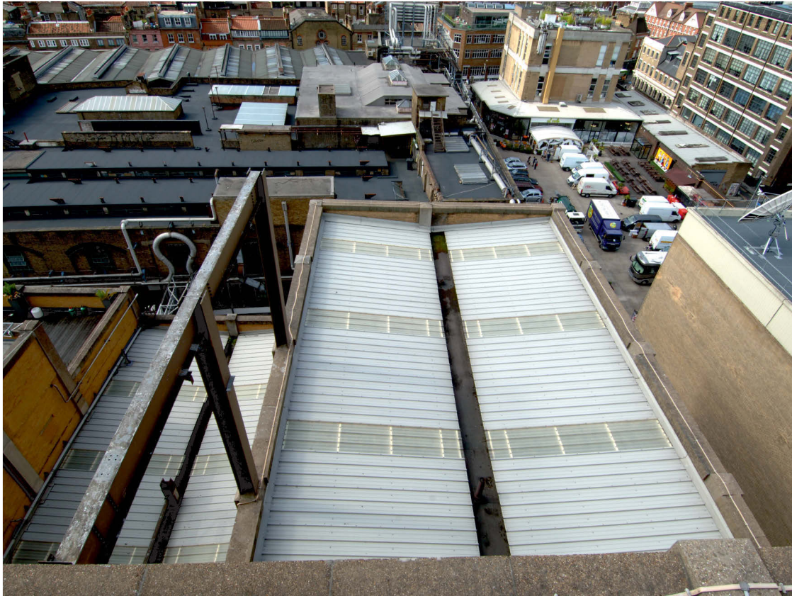
Fig 14 The roof of Area 1, viewed looking south from the roof of Area 3
