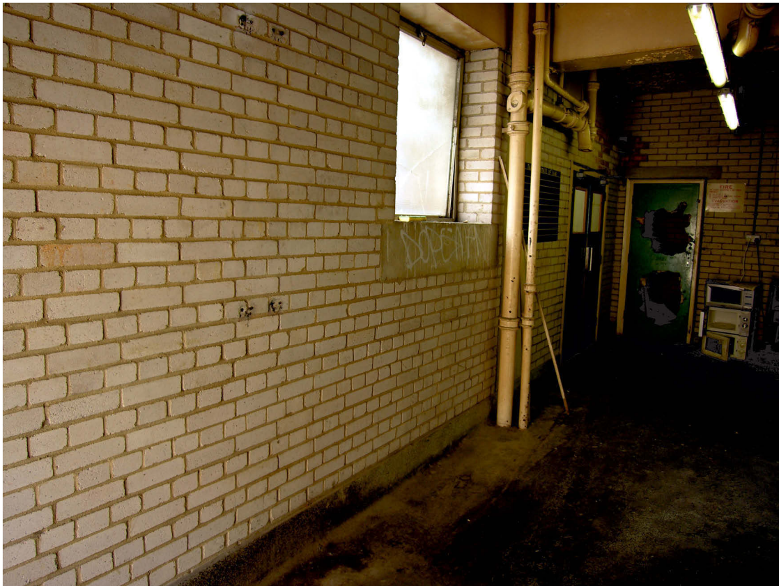
Fig 26 The English bond brickwork in the east wall of Area 3, 4th floor, looking south
