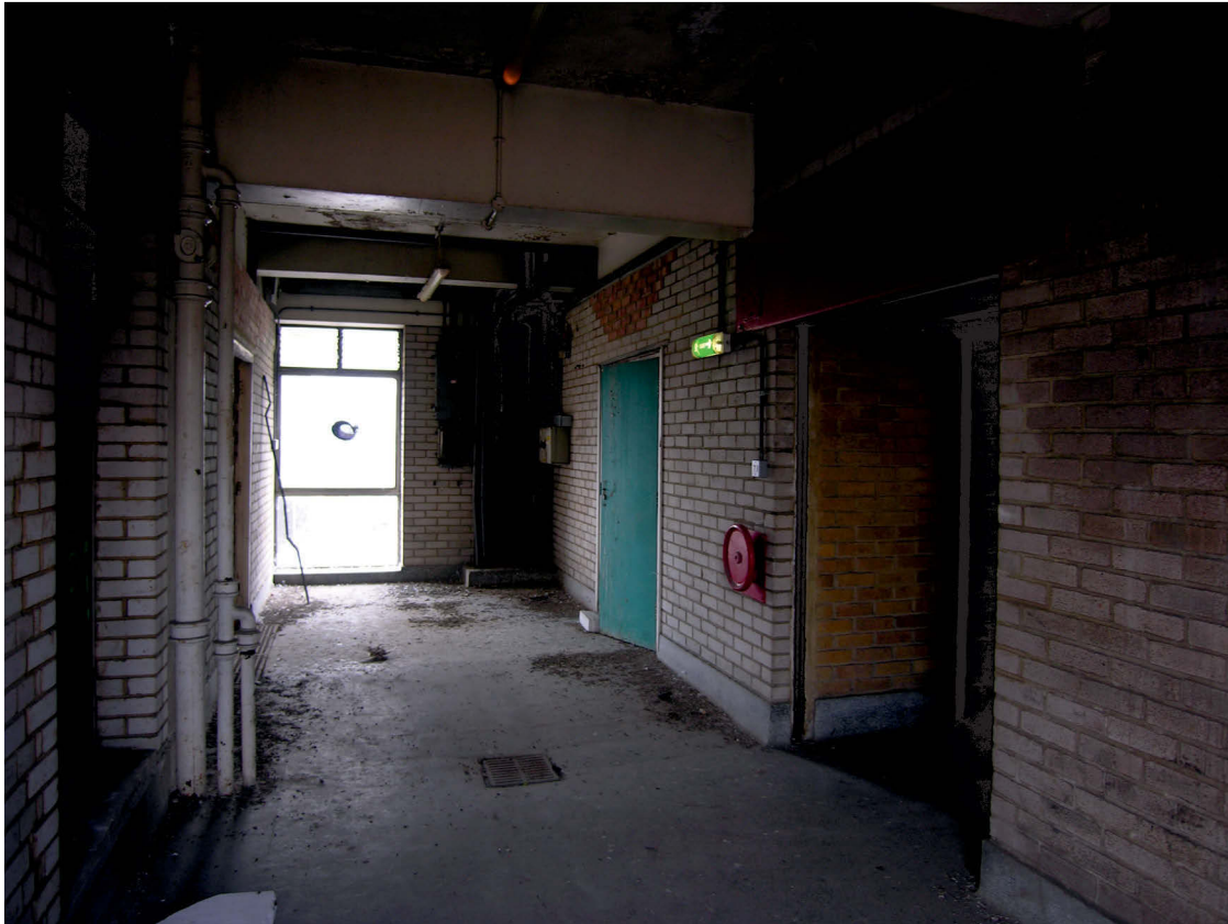
Fig 24 The lobby area of Area 3 with the rolling shutter fire door, looking south
