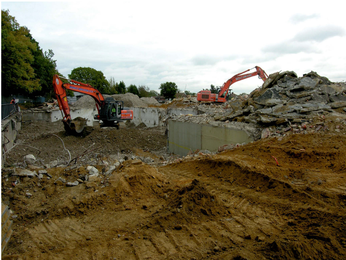
Fig 4 View of boiler room in Pitch 2 from west
