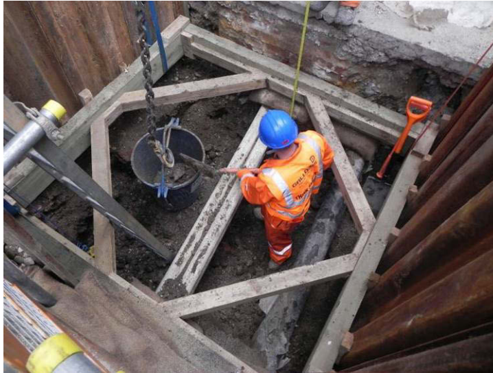
Photo 9: Pit 2 – Galldris excavate 19th and 20th-century utility and construction backfills, looking south-west.
