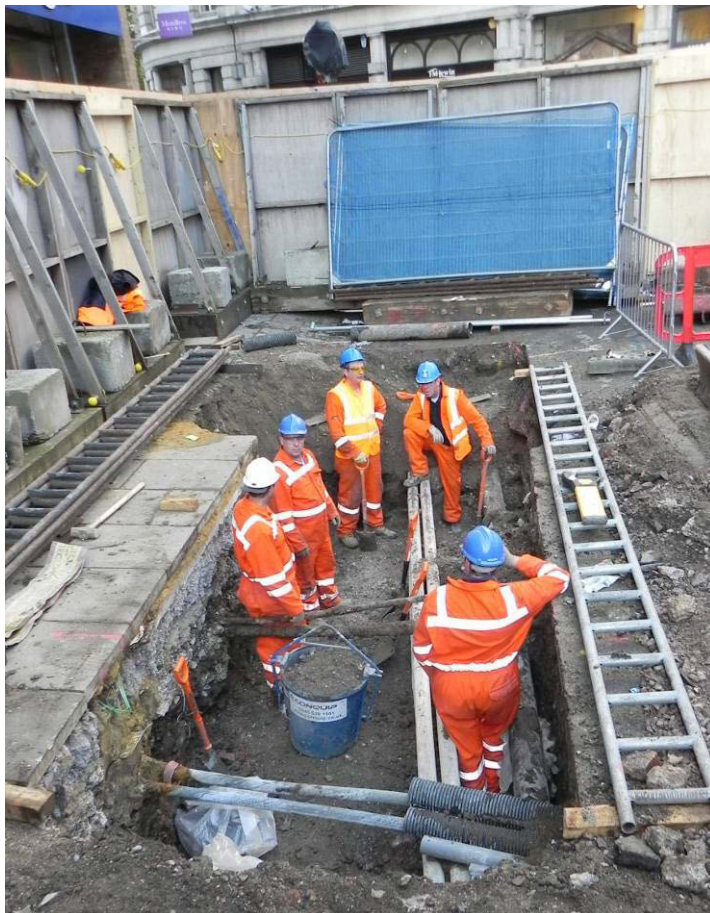
Photo 10: Pit 3 – Pit location, showing excavation of modern overburden with utilities, looking west.
