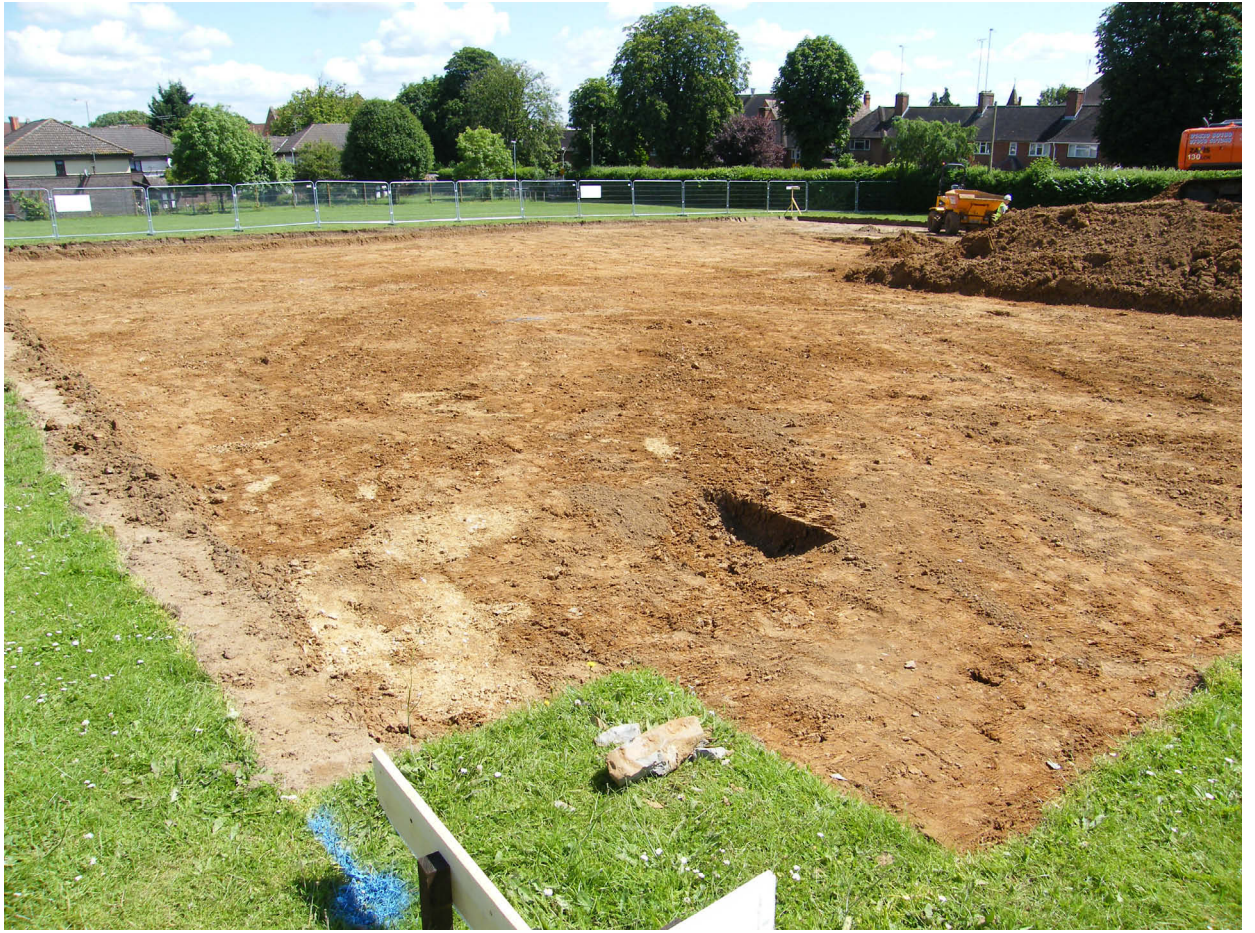
Fig 3 Photograph of strip, map and sample investigation area looking north-east showing excavated slot across natural feature [2] in Area 1
