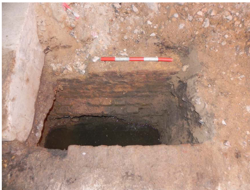
Photo 1, Brick foundation for platform [76] (top of picture), railway foundation [77] (base of picture), looking north.
