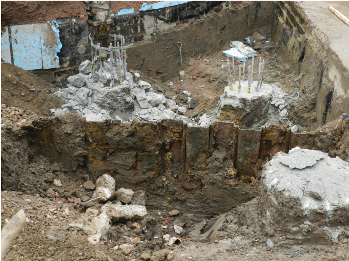
Fig 4 Crane base trench; piles and maximum depth of trench excavation (looking west)
