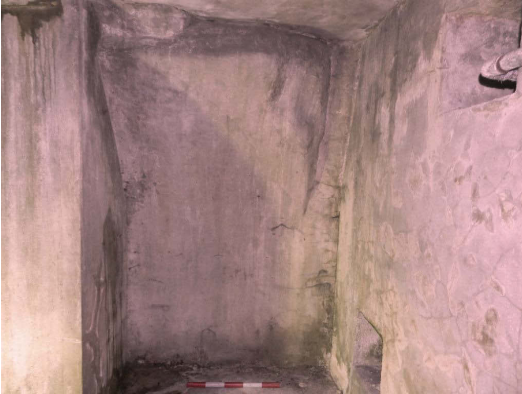
Fig 18 The east end of the southern vault, looking south, showing broken south wall (MOLA image 14)
