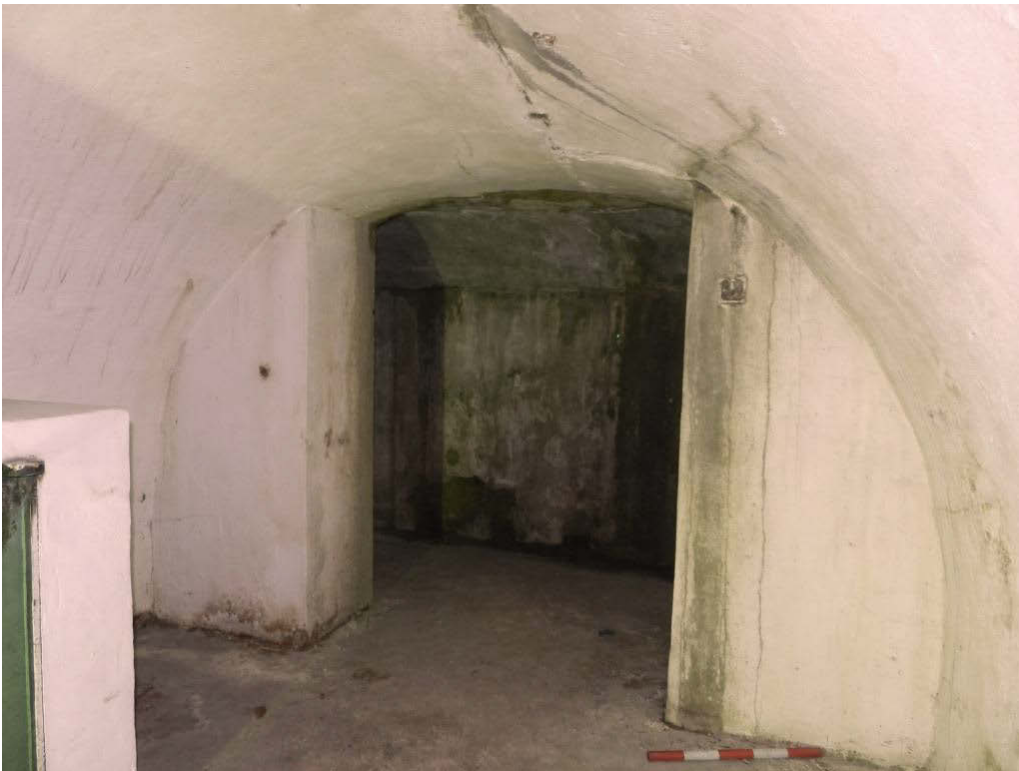
Fig 15 Connection between the northern vault and the half-vault, looking north-east (MOLA image 25)
