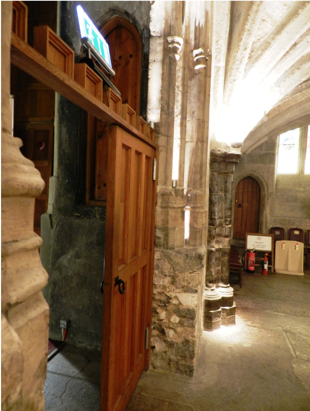
Fig 8 View of the south jamb of the east door to the East Crypt, looking south-east. Note the door to the garderobe stair within the thickness of the jamb, the difference in floor level between the ground and threshold of the garderobe stair and in the background the door to the south-eastern stair turret.
