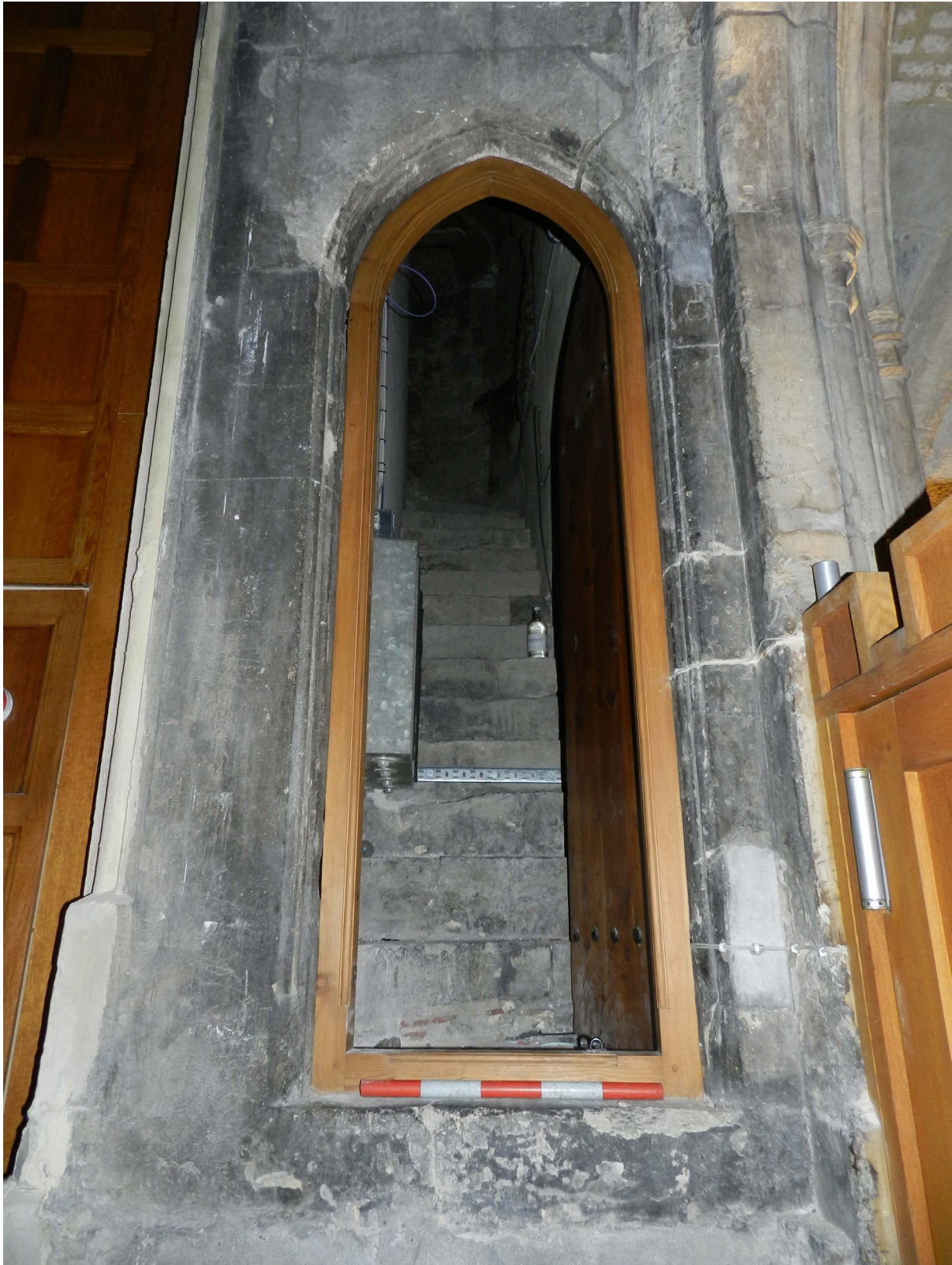
Fig 15 Intra-mural garderobe door and access stair within the south jamb of the east door to the East Crypt, looking south
