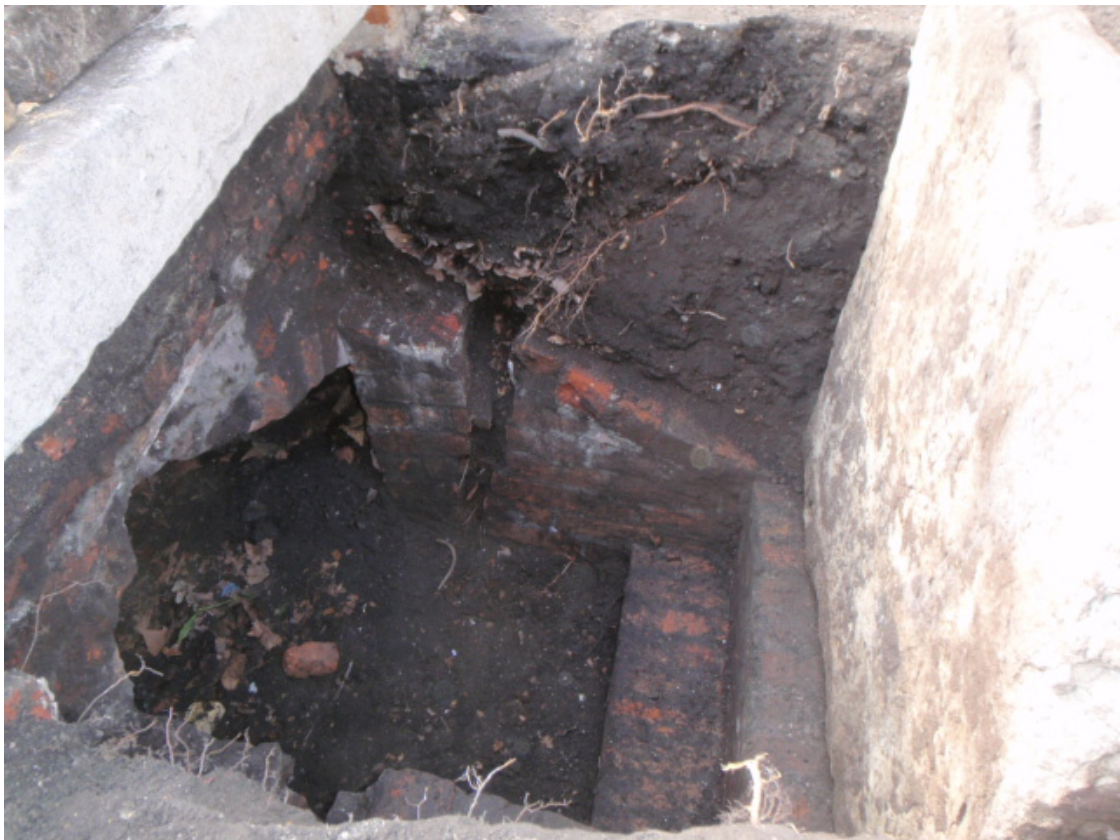
Fig 4 The entrance to tomb 119, looking south. Note the crack in the south wall (opposite) and the missing bricks of the vault crown (to the left).
