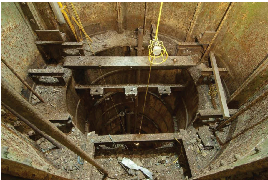
Fig 12 Remnant equipment at the bottom of the upper part of the well (08512027)
