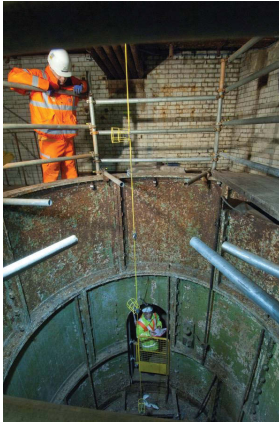
Fig 11 The upper part of the well and the inspection door, looking east (08512024)
