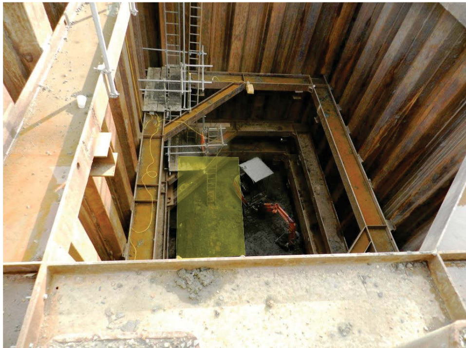
Photo 3 Ham Sewer Access shaft, late 19 th - or early 20 th -century culvert at 96m ATD as highlighted in yellow
