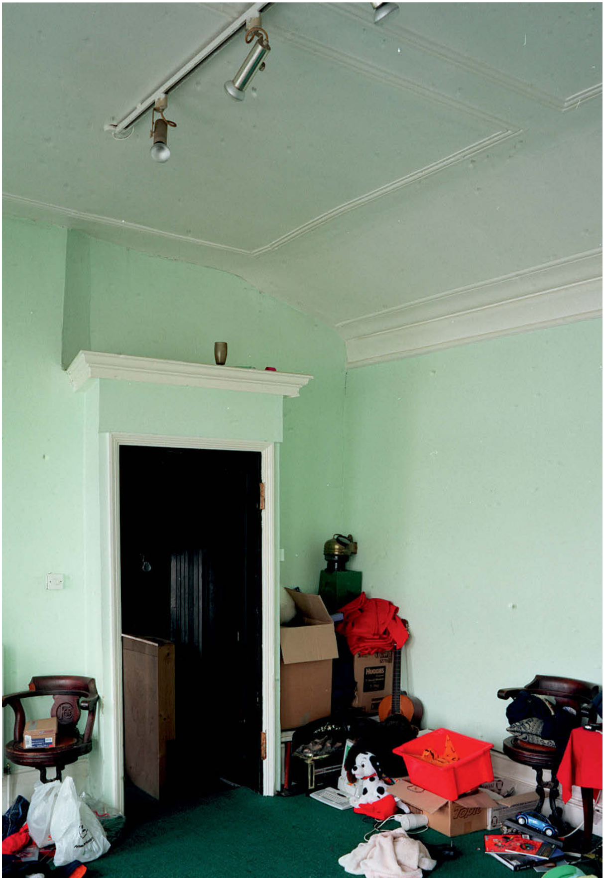
Figure 18. The interior of a late eighteenth century first floor dining room in The Gun, Room 1FI, looking south-west to its entrance porch above a spiral staircase (MoLAS 387/01/15)
