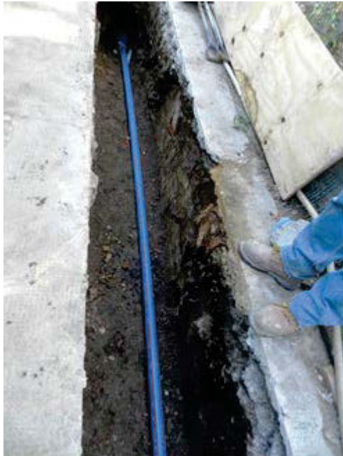
Photo 12 Trench on east side of king John Street (site entrance) in the pavement
