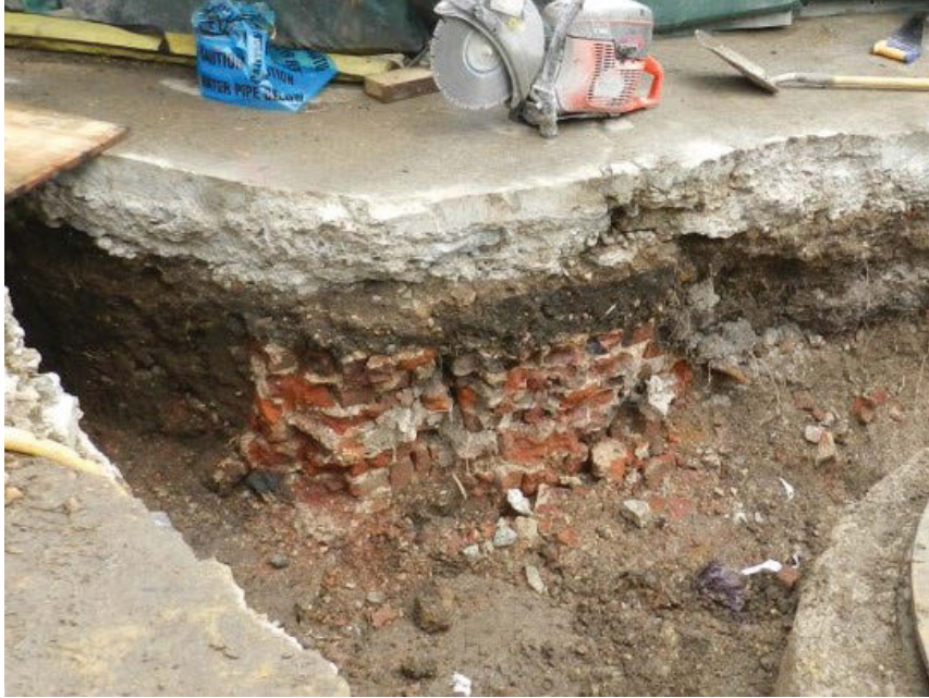
Photo 9 Wall made from Tudor-style 2-inch thick bricks east side of new manhole
