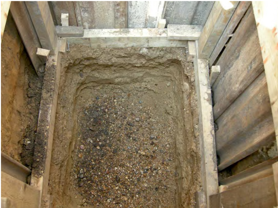
Fig 9 View of Trench 2, looking west, with natural gravel shown in the base of the trench
