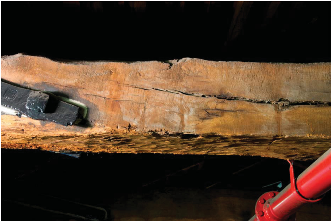
Fig 11 Detailed photographs showing the south end of the Truss 9 tie beam with its sawn side axe hewn lower face
