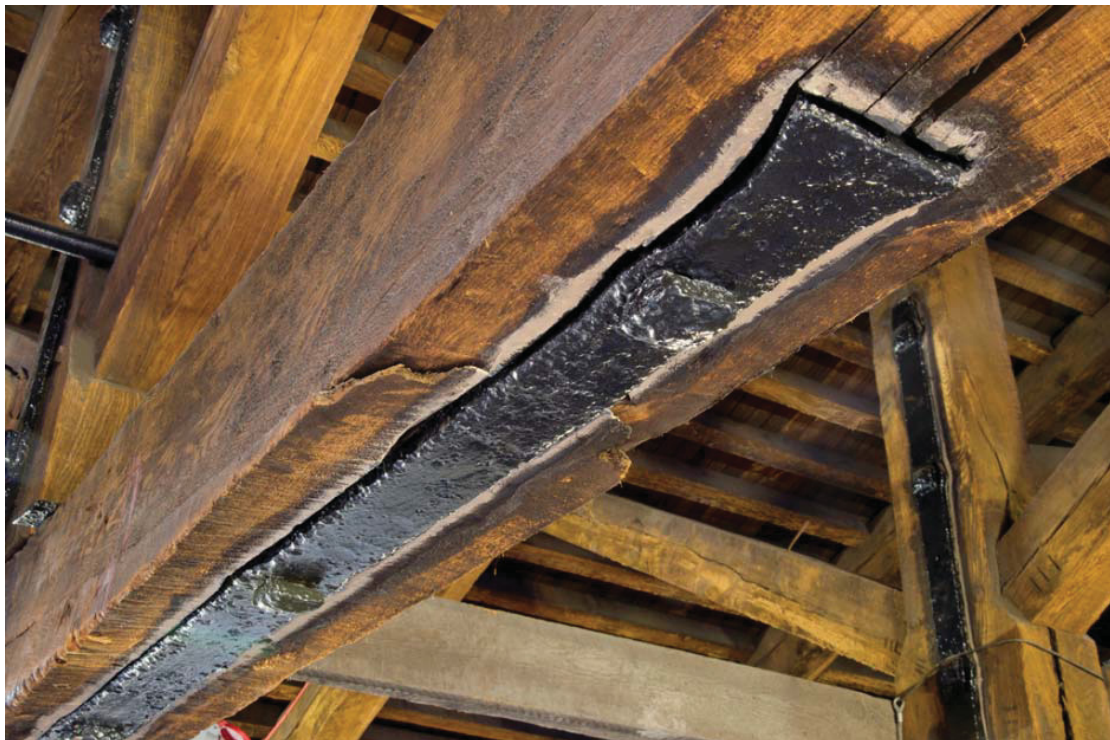
Fig 13 Photograph showing details of the simple through splayed scarf and original inset iron reinforcing strap, in the soffit of the tie beam of Truss 20. Shows how recessing of the dovetail ended iron strap was crudely done with a slack fit and cutting away of the ends of the scarf joint. The paint is modern
