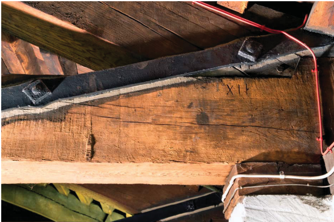
Fig 12 Detailed photographs showing of Truss 9 looking west, shows a ridge left where sawing out the face from both ends converged but did not quite meet, probably indicative of sawing on two high trestles. Also showing a combined joint and truss number cut with a 2" chisel and given a 'tag'.
