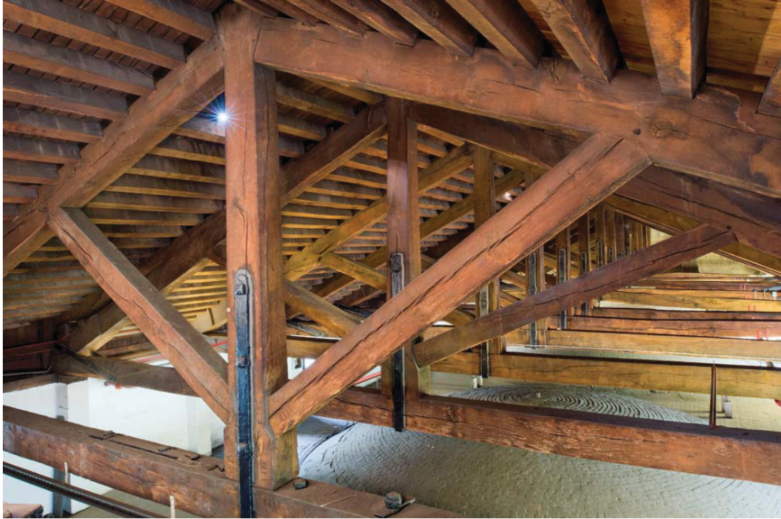
Fig 5 General photograph of the form of the horizontal tie beam roof trusses of St Pauls nave central roof looking east with Truss 14 in the foreground. Showing part of the through splayed bolted scarf in the, slightly wider, western, Truss 14 and the unscarfed 14.08m (46' 2") long tie beams used in the eastern trusses. Also visible are the chisel cut, combined truss and joint numbers in 2" and 1" sizes.
