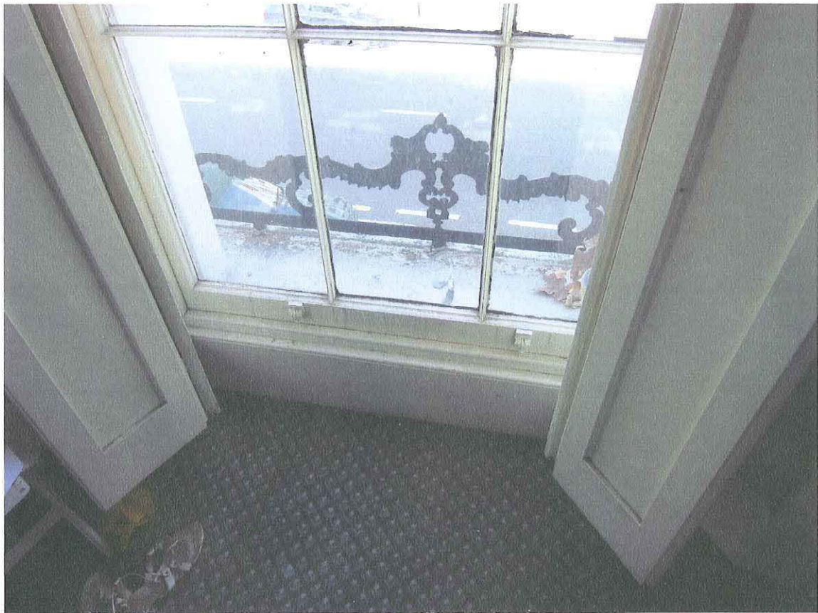
Fig 8 Detail of 1st-floor front window shutters, sill and pot-guards, looking east (MoLAS)
