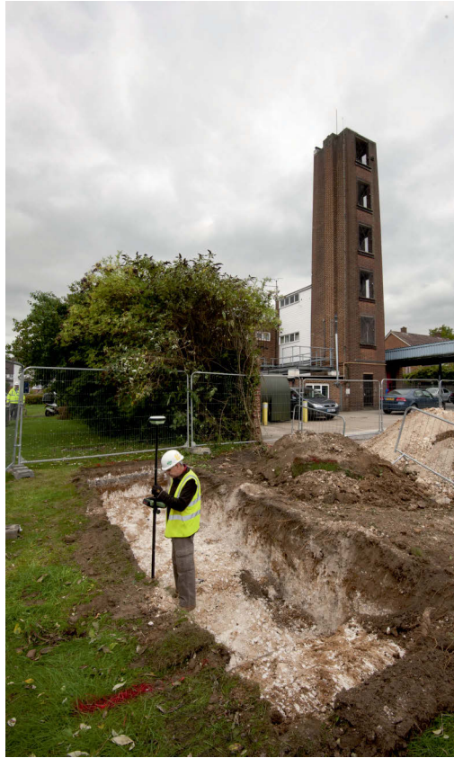
Fig 7 Photo of Trench 5 (looking south-west) showing a member of the MOLA Geomatics team using GPS to locate the trench
