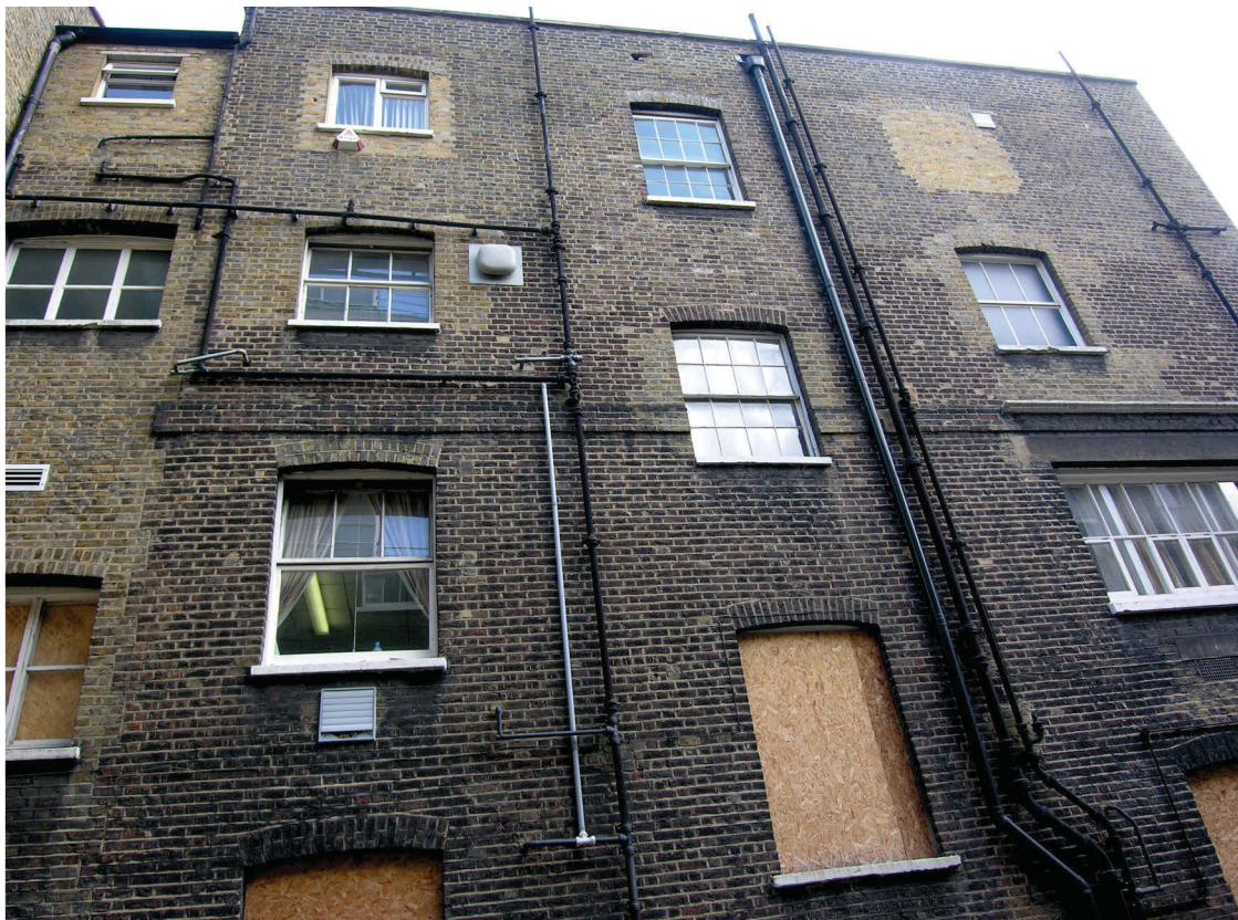
Fig 13 North wing of the 18th-century building, north elevation, showing junction with later additions (left) and original or early 8-over-8 sash windows on upper staircase landings
