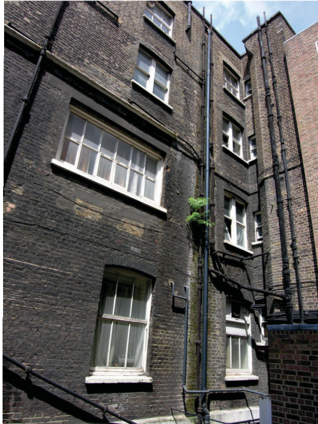
Fig 12 South wing of the 18th-century building, south elevation, showing junction with later additions (right)
