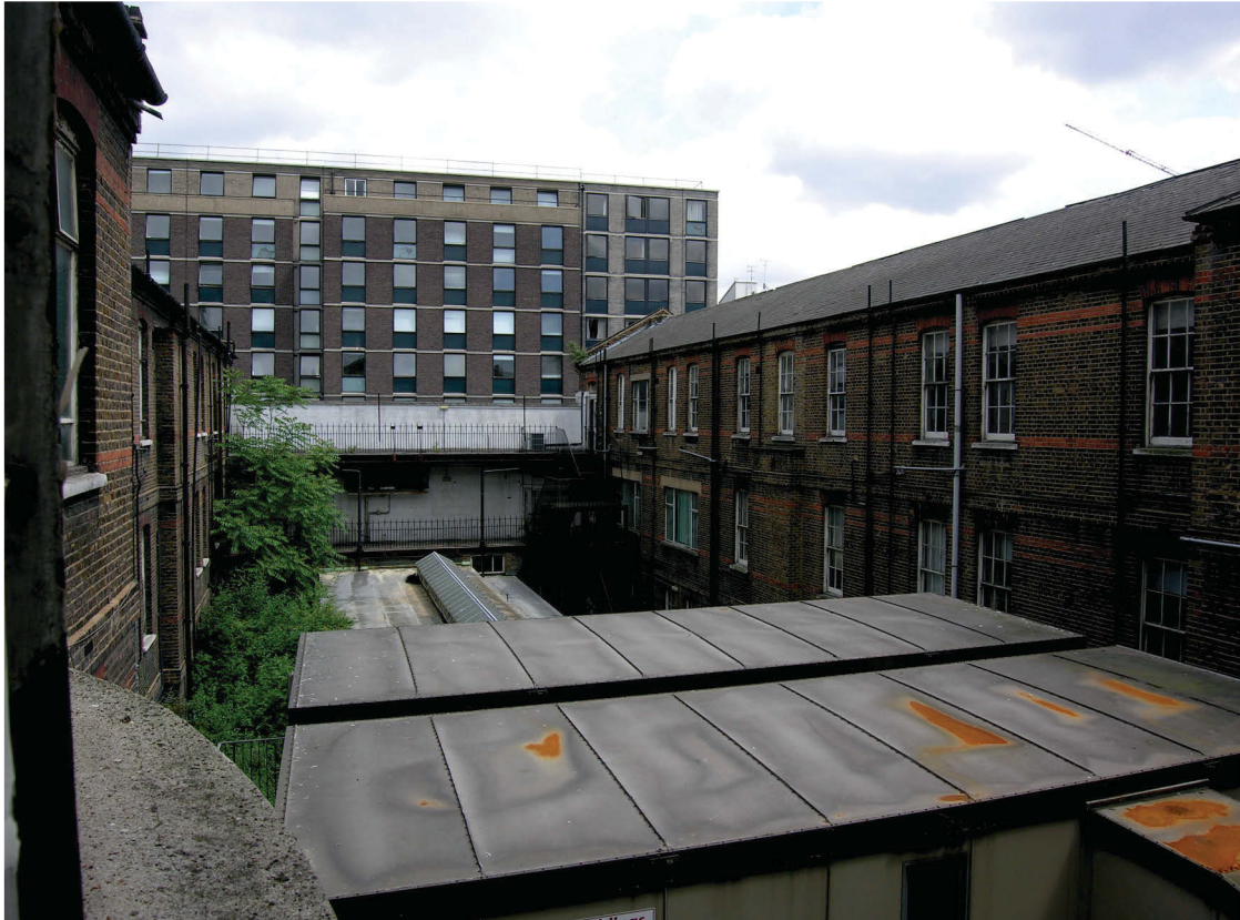
Fig 20 Open galleries against high boundary wall at east end of site, closing off central yard
