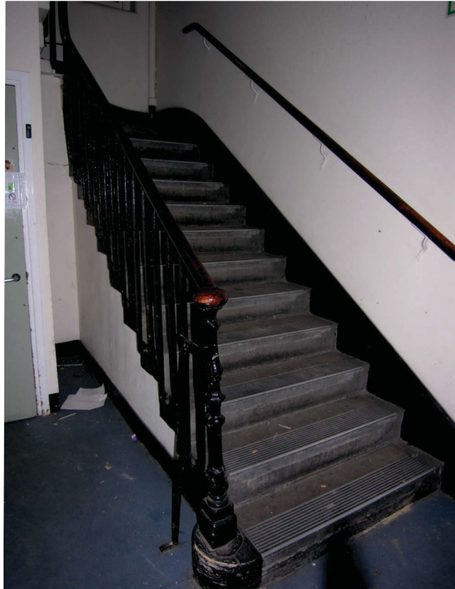
Fig 16 Staircase in north wing of 18th-century building: stone steps from basement to ground floor, and wrought-iron balusters
