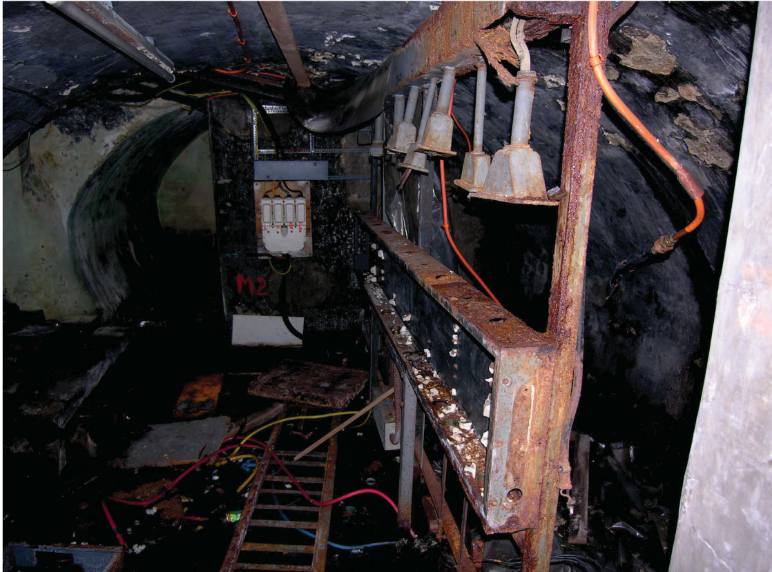
Fig 14 Vaulted cellar under forecourt of 18th-century building, with 20th-century electrical switchgear
