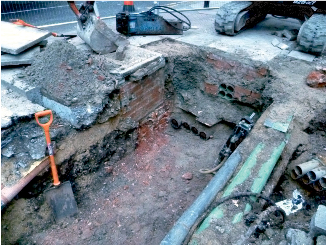
Fig 3 Watching brief Trench 1, looking east. Shows remains of 18th-century brick wall beneath modern brick manhole
