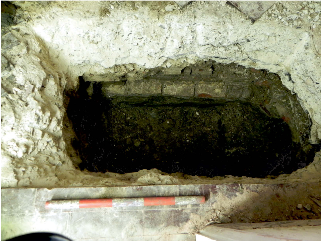
Fig 3 Photograph of evaluation trench 1 showing the remains of part of early Victorian wall, relating to the building that predated the present one (looking north)
