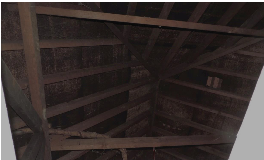
Fig 30 A view into the loft from the hatch in the first-floor hall
