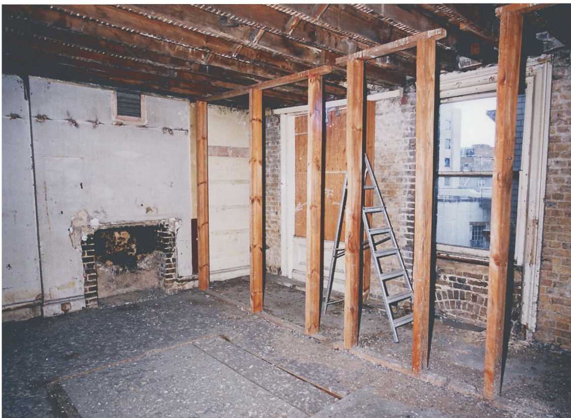
Fig 49 4F9/10, covered void for lift shaft in the foreground. Looking north-east (Tweeds 04/176)
