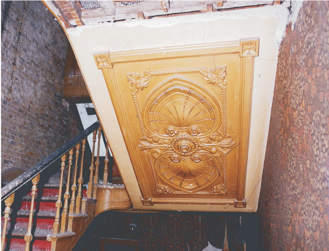
Fig 36 2F17, detail of plaster decoration on underside of staircase leading to 4th floor (Tweeds 04/151)
