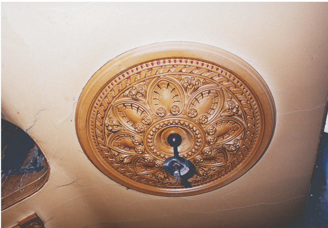
Fig 37 2F17, detail of plaster ceiling rose on landing between 2nd and 3rd floors (Tweeds 04/153)
