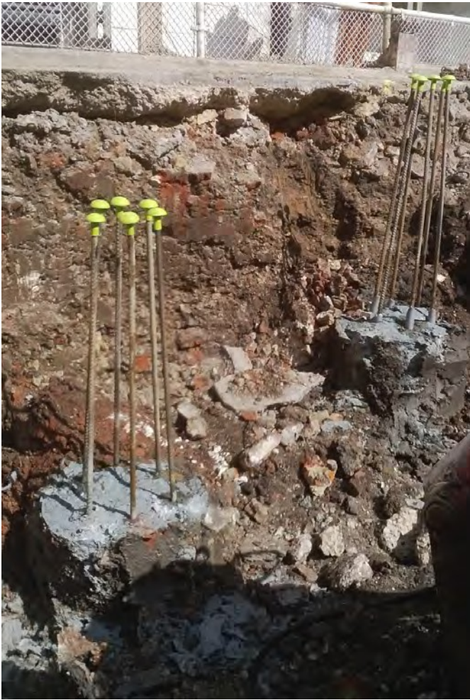
Fig 12 Photograph showing typical pile cap at east side of site (pile cap 13), view to west
