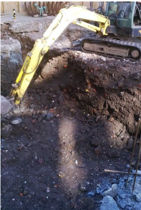
Fig 11 Photograph showing typical pile cap at west of site (pile cap 5), view to east
