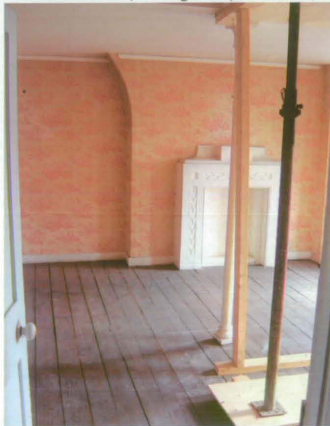
Fig 45 Fire surround in 3F5 and steel column inserted, probably after the north wall of this room was moved northwards; looking east. The steel column has been reinforced recently with acrow props (A J Browne, Architects)
