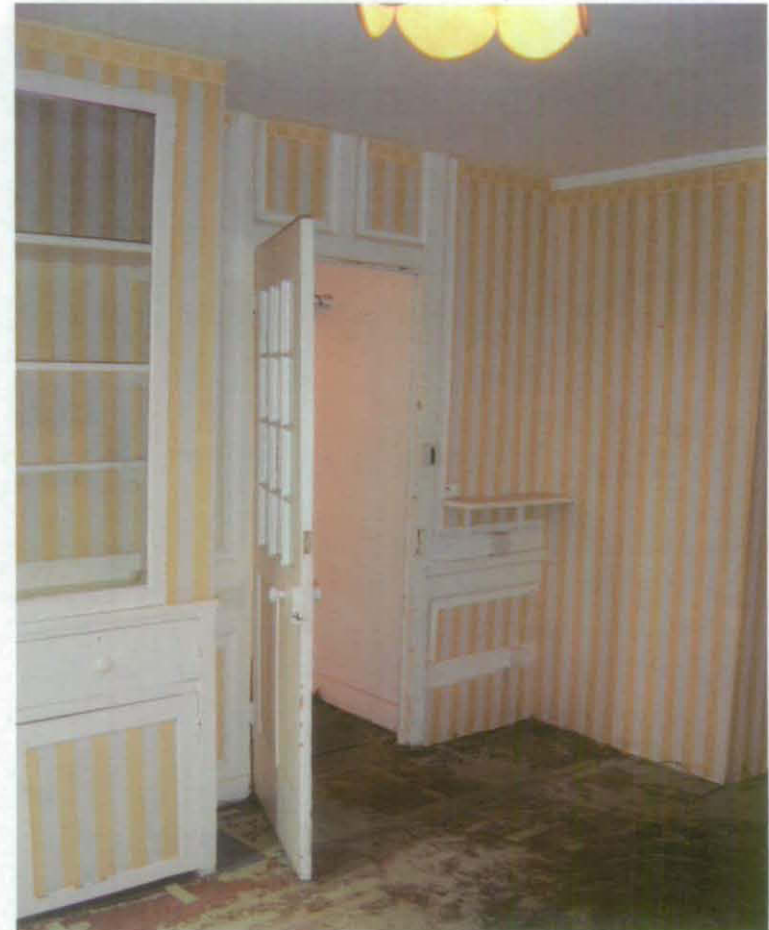
Fig 37 High-quality panelling [15] inserted to form a new west wall in the former kitchen, dividing B16 from a passage beyond, B17; looking north-west. The panelling is too large for its present position and was perhaps taken from elsewhere in the house. The dado rail has been shaved to allow the glass-panelled door to swing flat against this wall, suggesting that the dresser was added to the wall later (A J Browne, Architects)
