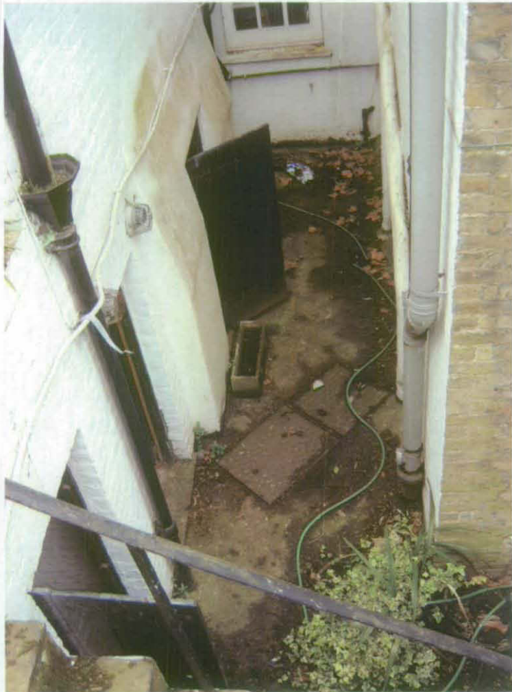
Fig 36: Rear basement yard B8, looking south, showing brick reinforcement [65] of the external face of the east rear wing (A J Browne, Architects)
