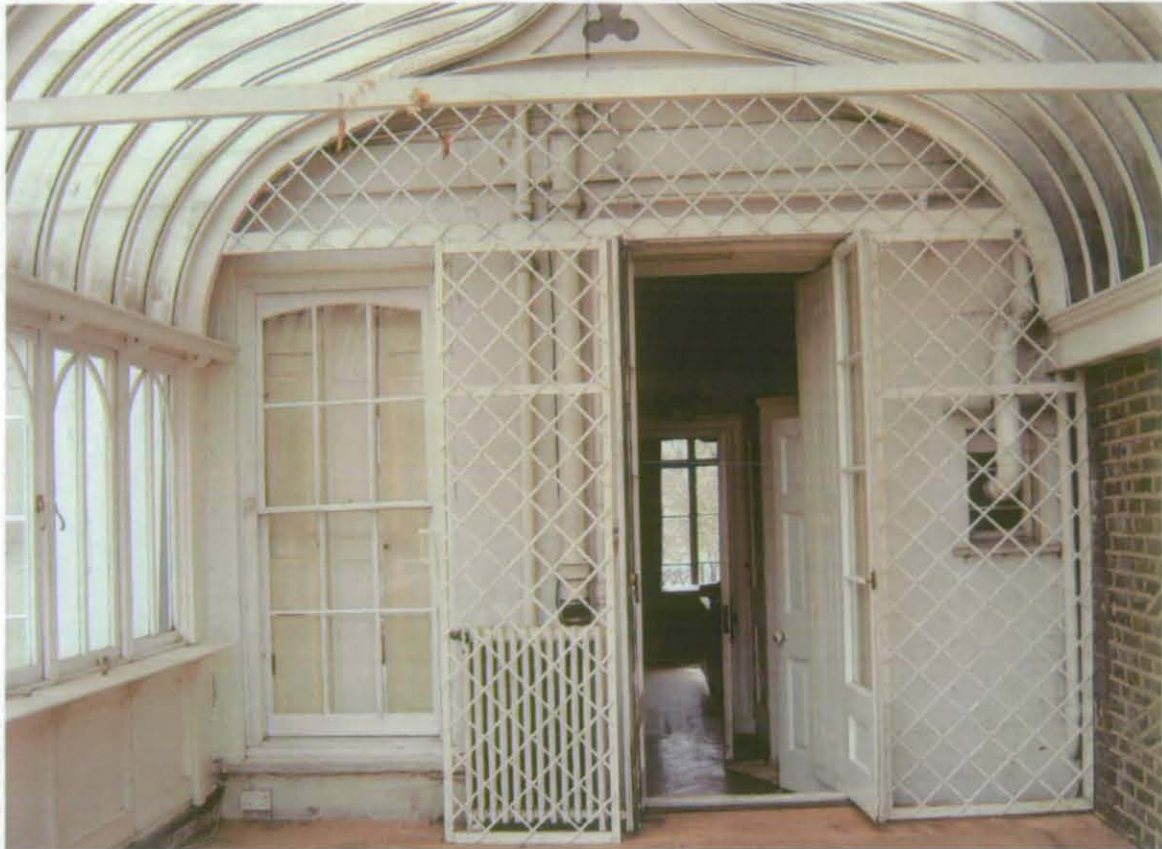
Fig 42 Functioning window and former window remade as a full-length doorway opening on to the flat roof of the west rear wing, with a small window inserted for a new WC; looking south. The plat band on the rear wall of the house, at 2nd-floor level, resembles that on the front at 1st-floor level. The prefabricated aluminium and PVC conservatory was added later still (A J Browne, Architects)
