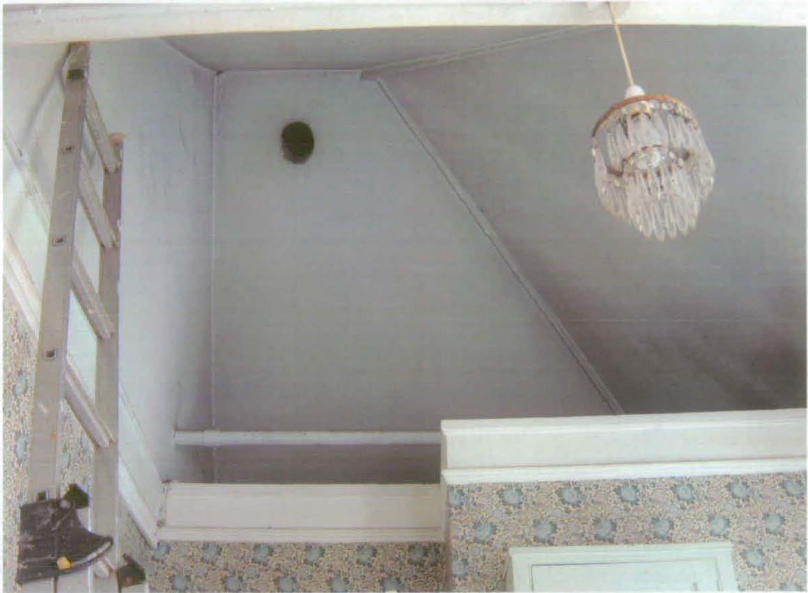
Fig 44 Ceiling of 3F8 raised to the full height of hipped roof R3, forming a higher-level space partly over rooms 3F6 and 3F7; looking west (A J Browne, Architects)
