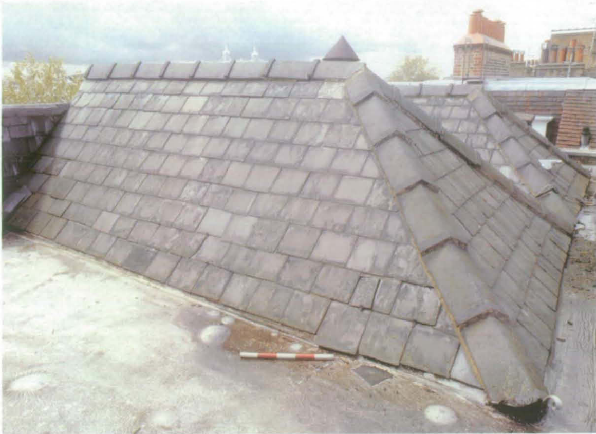
Fig 26 Hipped ends of two roofs running from south to north; looking south-west
