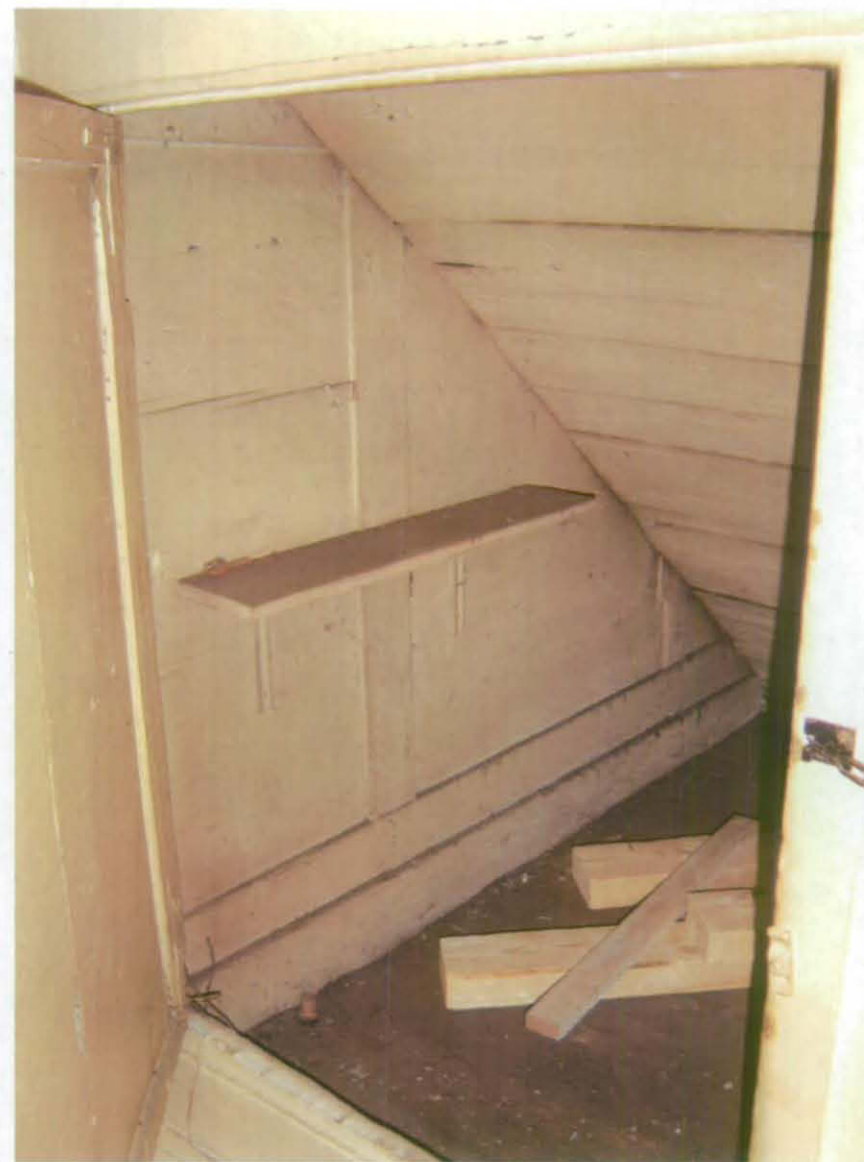
Fig 39 Plain panelling on the west wall of B18, probably original, underneath and predating the addition of service staircase [16] between G1 and B4; looking north-west (A J Browne, Architects)
