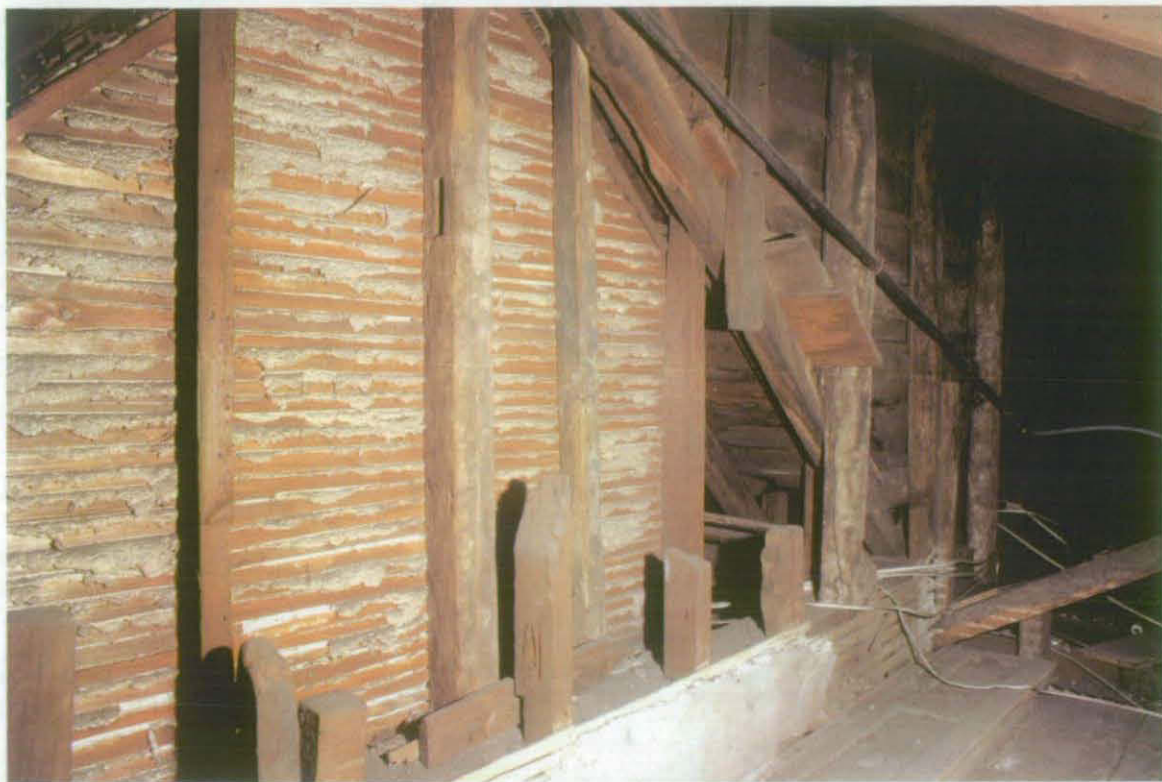
Fig 35 Inside the monopitch roof space of R1, looking north-east at the adjoining southern ends of two (formerly three) double-pitched roofs, R2 and R3
