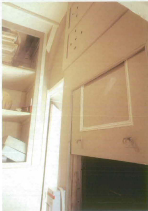
Fig 29 Isolated stair string [9] surviving above a door frame in G3, indicating the former existence of a staircase there between the ground and 1st floors; looking north-west. Hatch to later food hoist [17] in foreground
