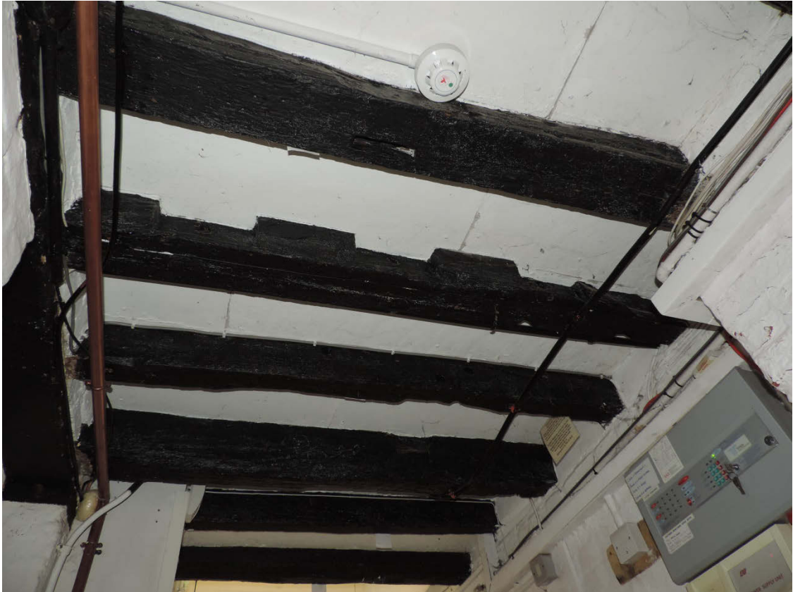
Fig 6 Timber [05], second from the top, showing multiple split mortises, facing east
