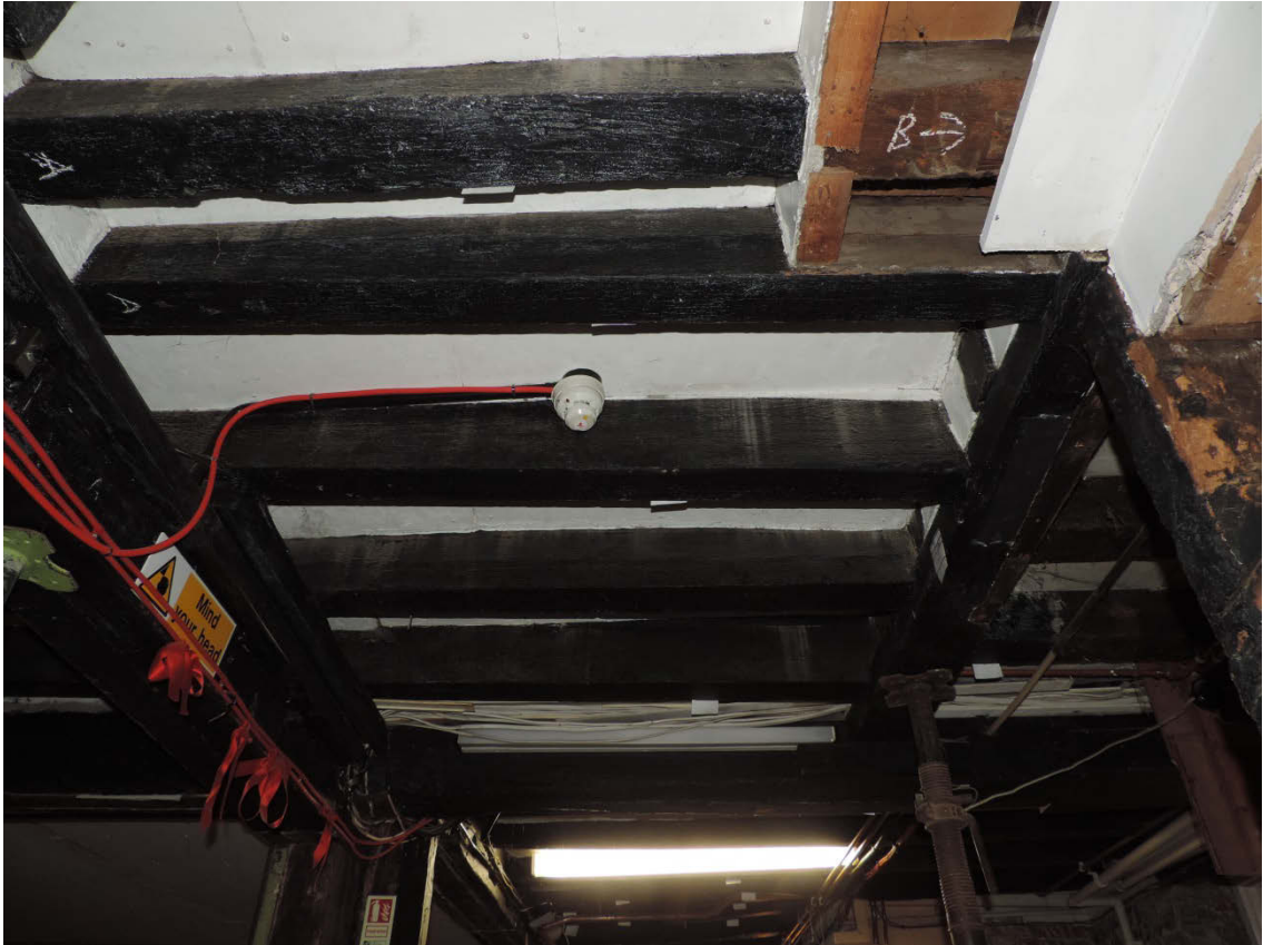
Fig 10 Recently added joists in area G, supported by modern bridging beam [103] and [104] to the left and right respectively.
