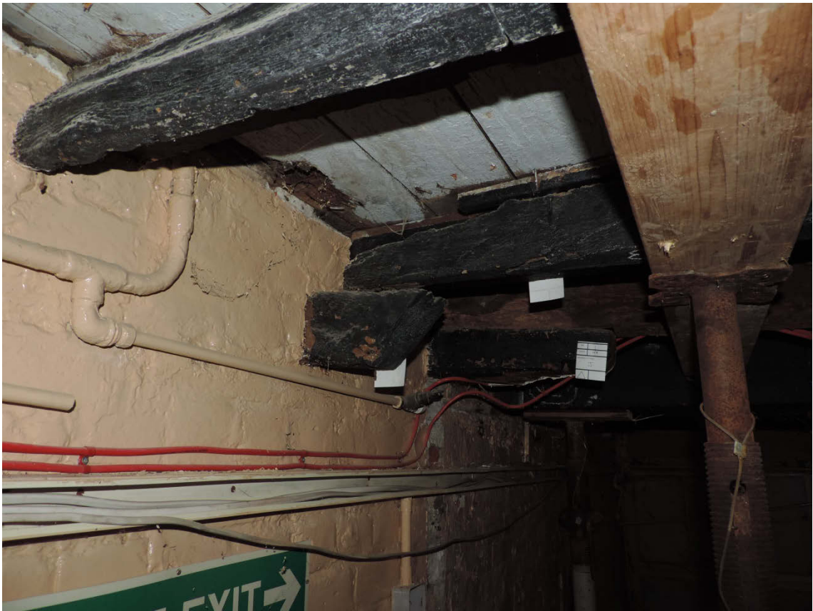
Fig 8 Showing a typical added corbel to support a joist likely too rotten at the end to stay within the wall.
