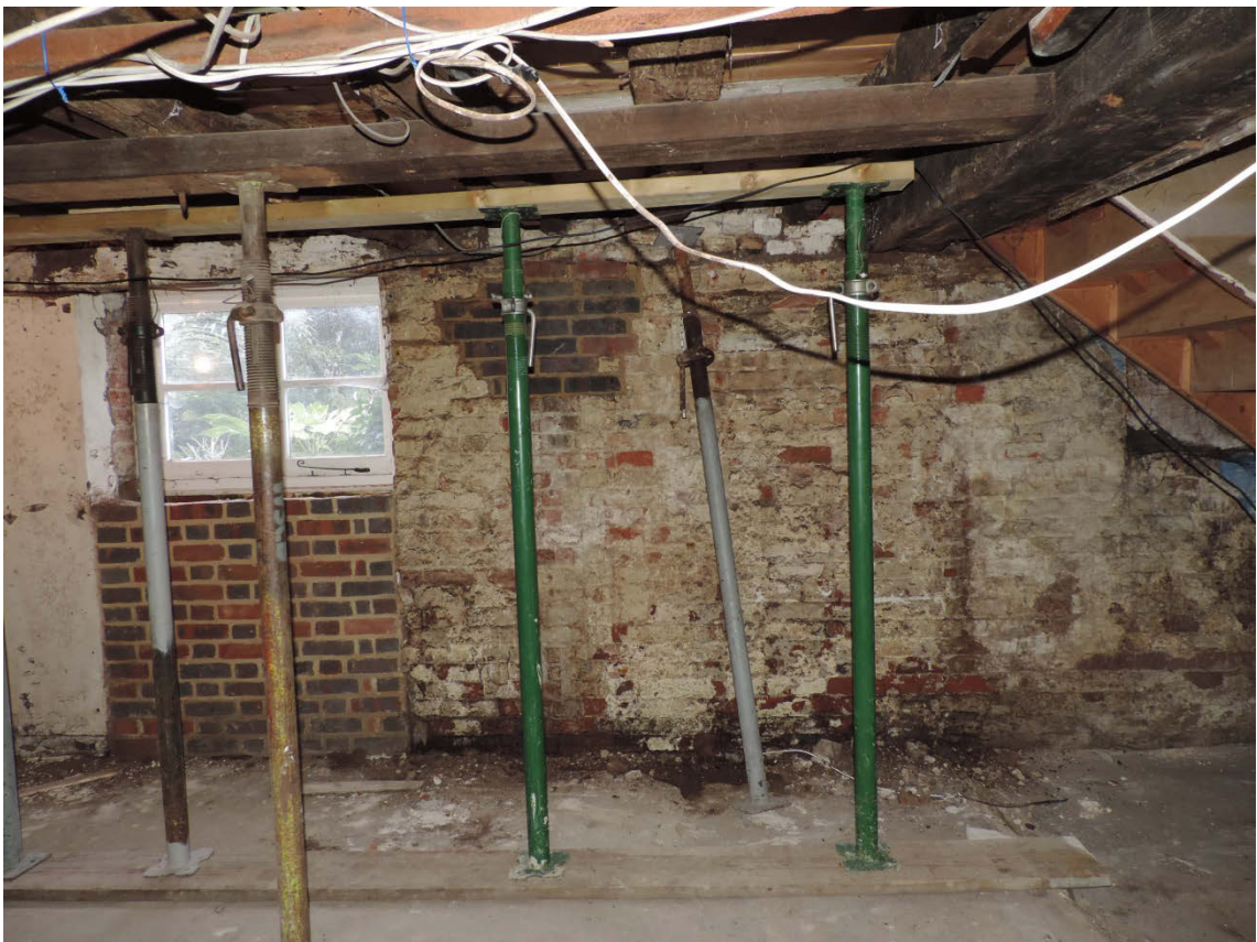
Fig 13 Showing the northern wall in Area K with several repairs and poor brickwork surrounding the timbers, facing north
