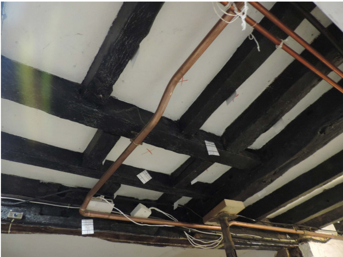
Fig 9 Area C arranged in a different pattern to the rest of the floor, likely to strengthen a weak area.
