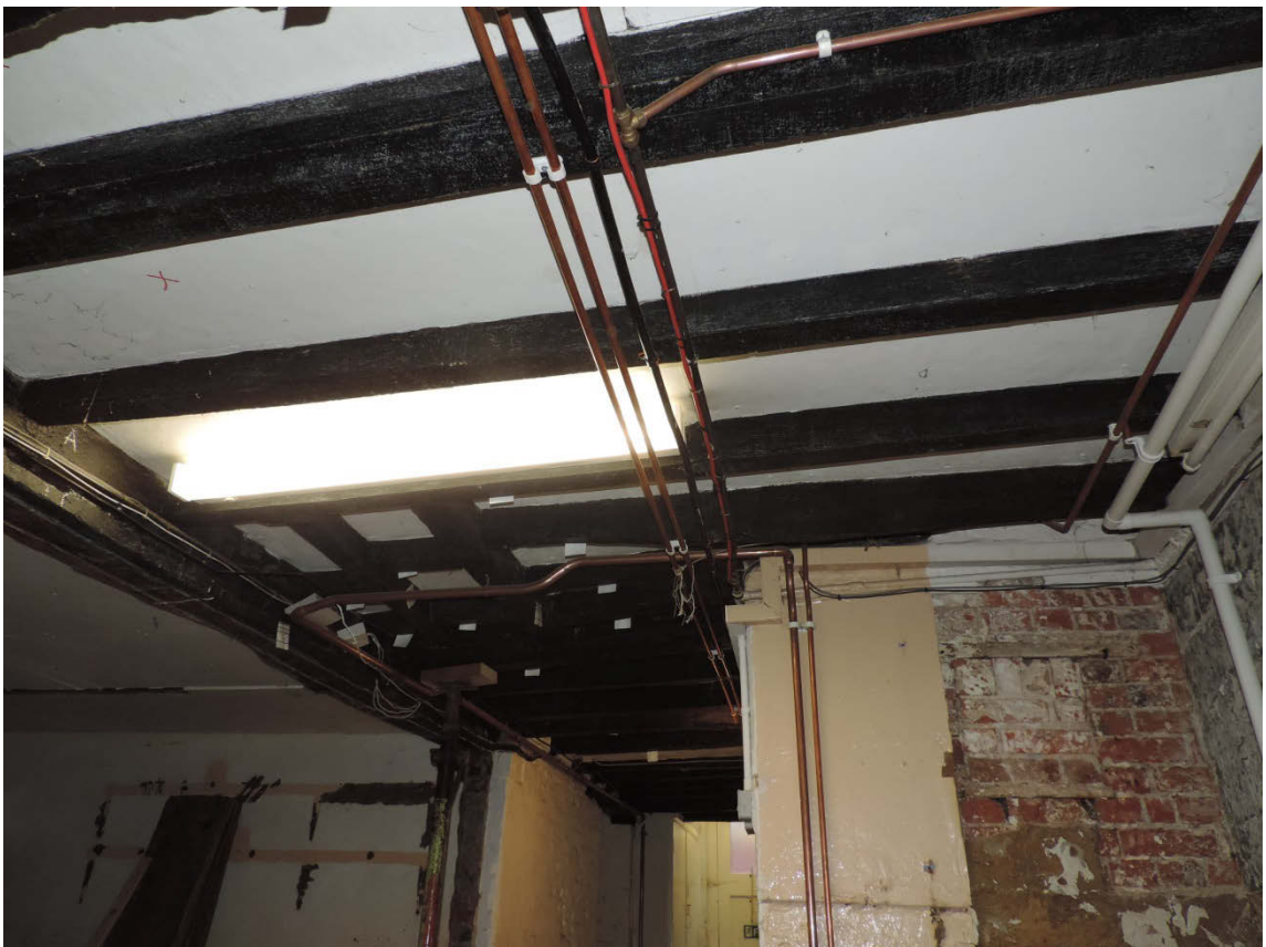
Fig 15 Showing the blocked opening along the southern wall in Area C, bottom corner of photo, facing east.
