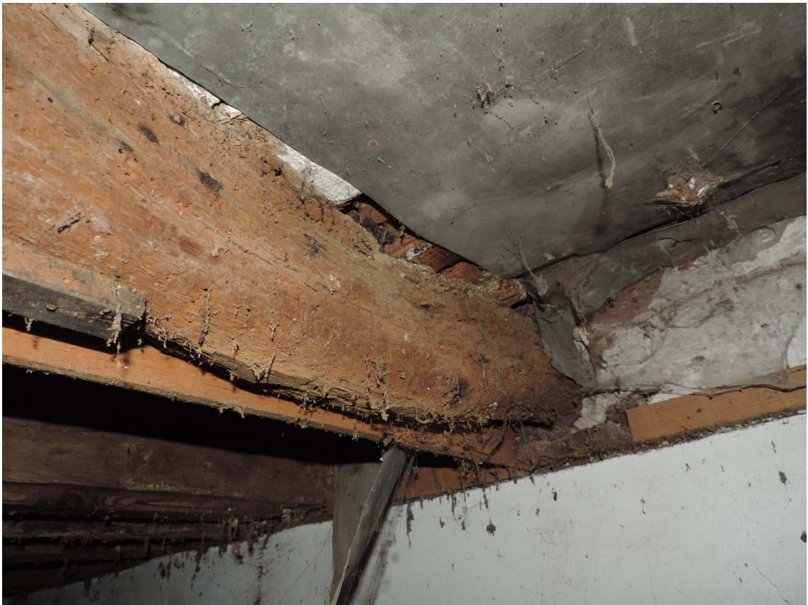
Fig 14 Showing typical decay where the timber joist inserts into the brick wall, facing north-west. Timber [70]
