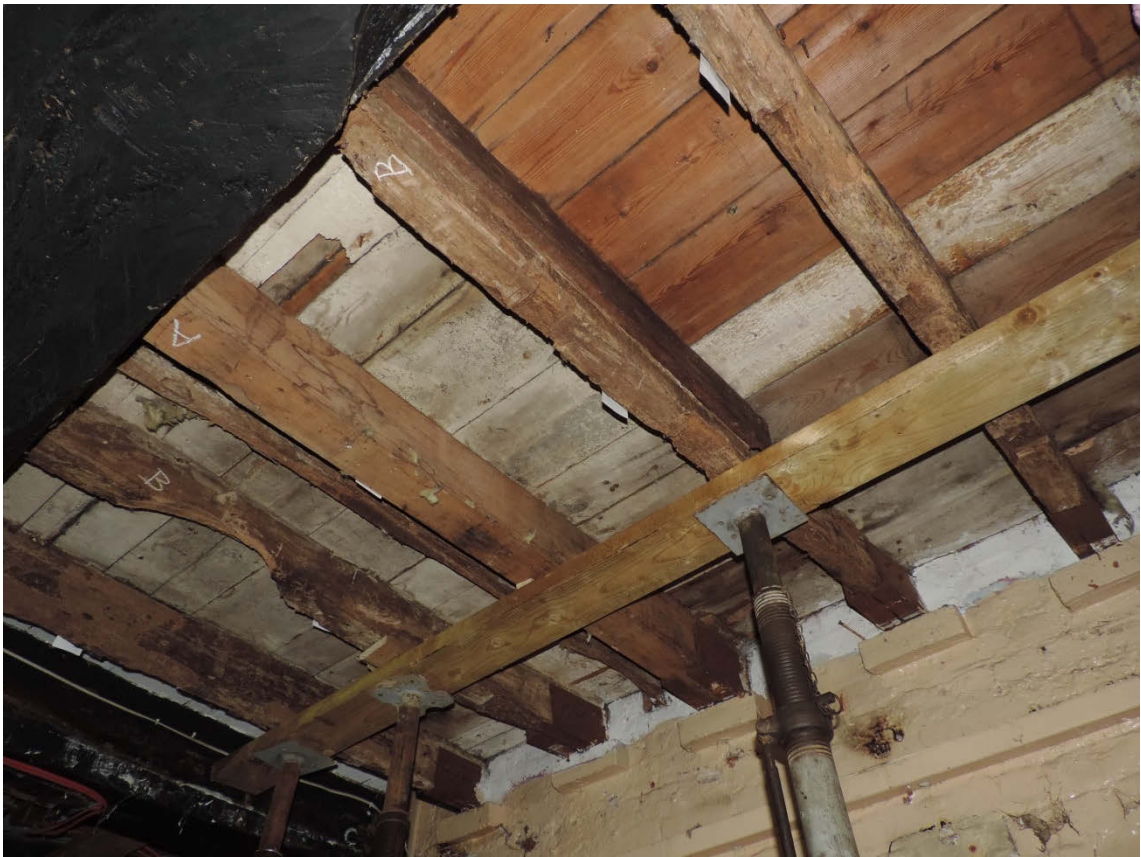
Fig 12 Area L, showing later added timbers and iron cradles supported by brick corbels.
