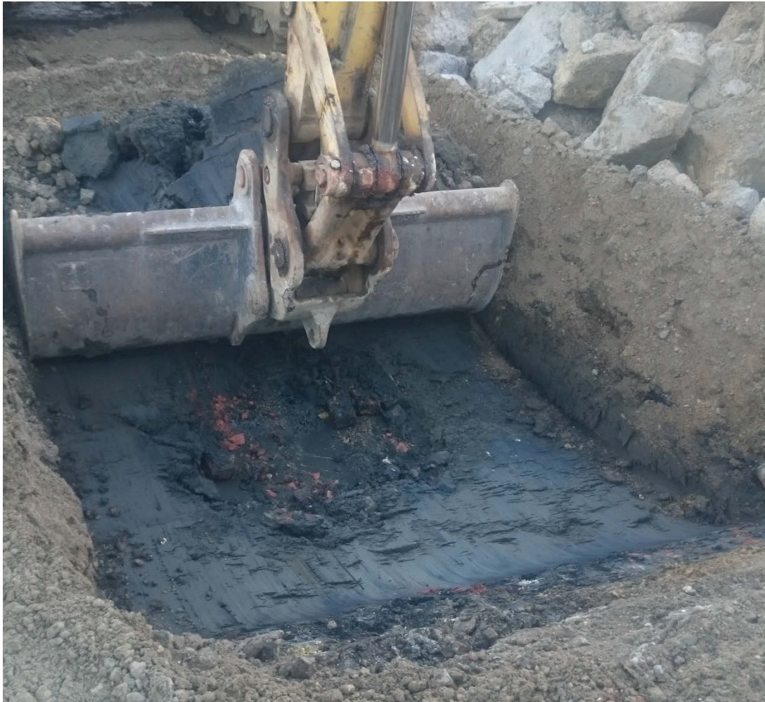
Photo 1 Trench 1, during excavation, London Clay is visible truncated by what appeared to be a manhole or soakaway, looking east.
