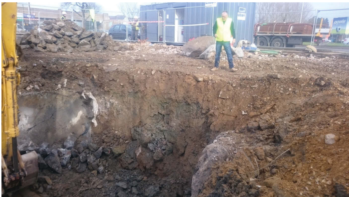
Photo 4 During removal of the concrete diesel tanks London clay was exposed in section beneath approximately 0.5m of modern material, looking north
