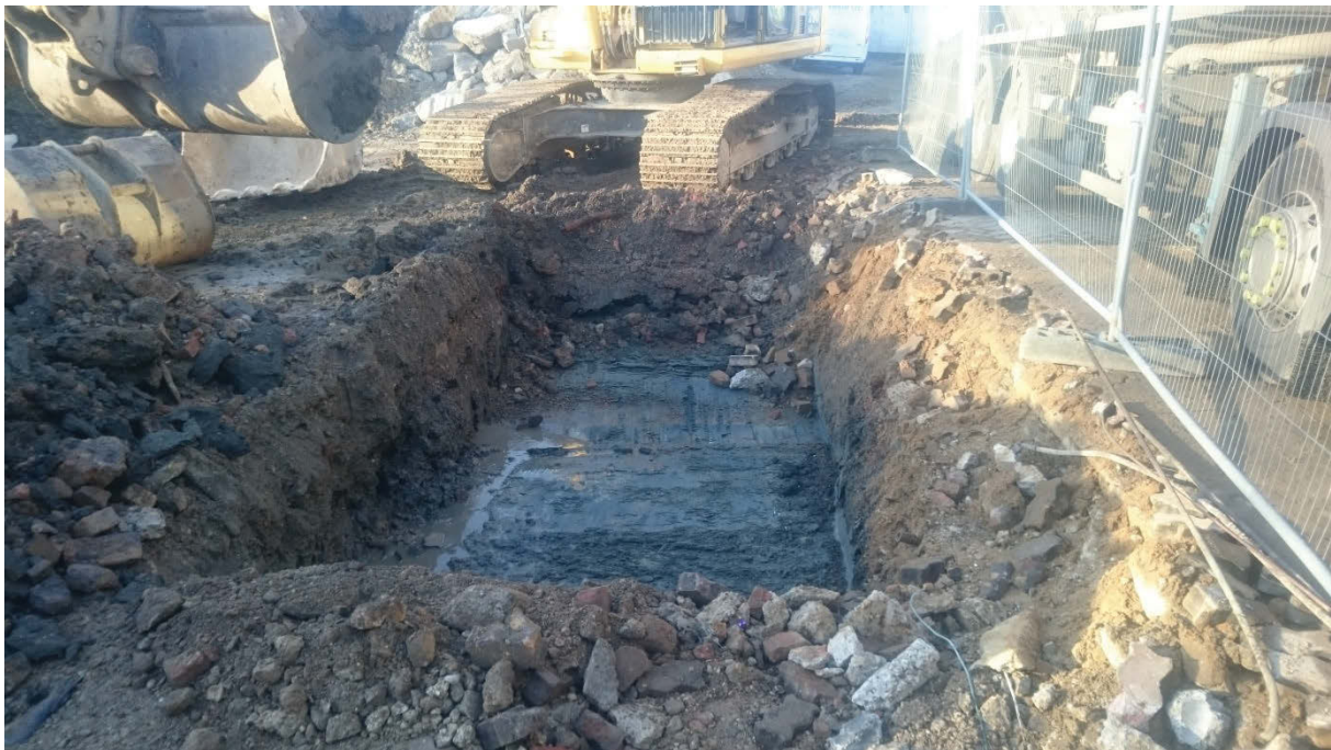
Photo 2 Trench 2, natural London Clay exposed across the trench base at c 24.50m OD, looking south-west.
