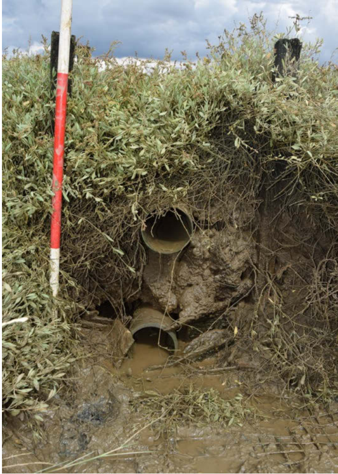
Plastic drainage pipes in northern end of north-eastern oyster pit
