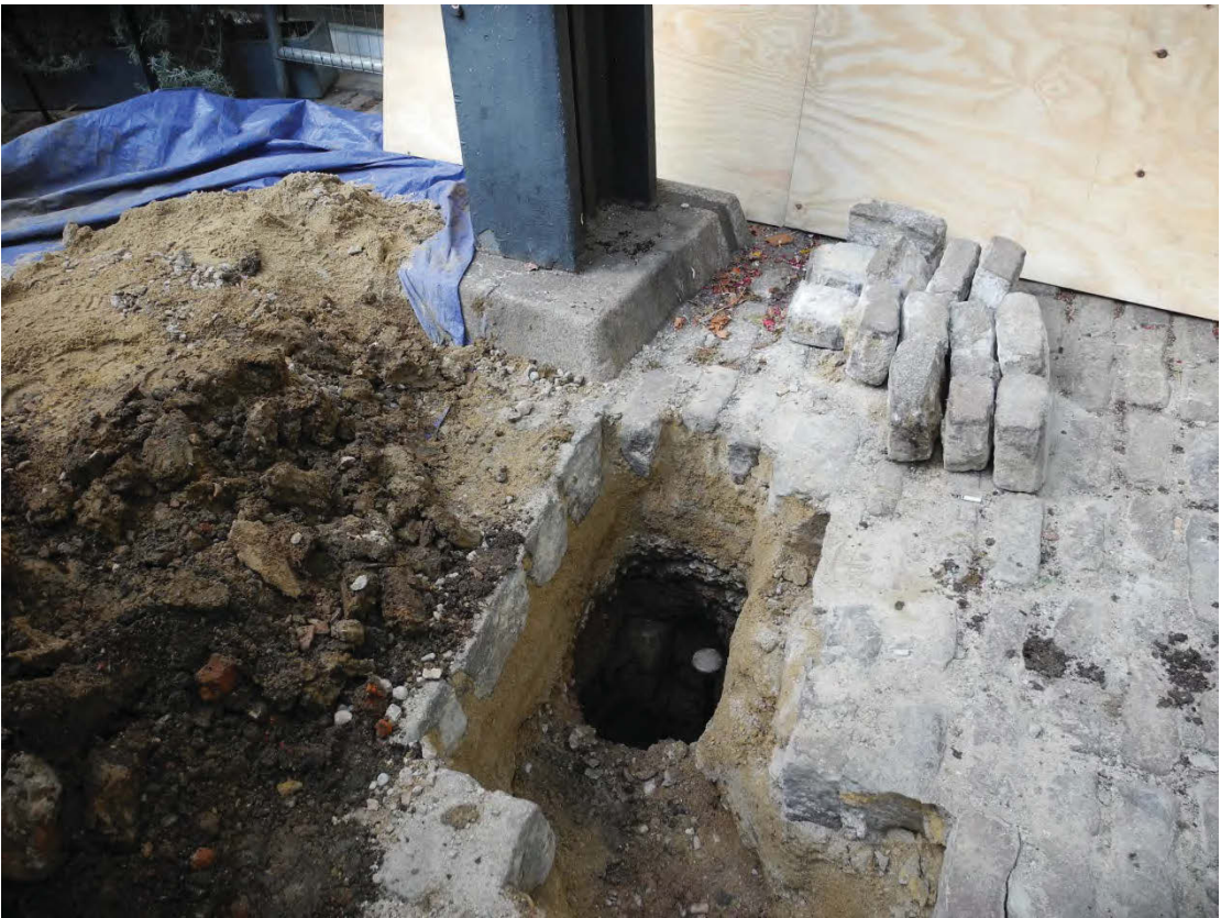
TP08 looking northwest, showing column, stone block is just visible in northwest corner of trial pit
