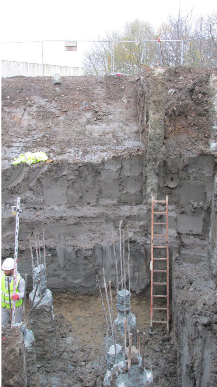
Photo 1: Plot A showing depth of alluvial clays over sands at the base of excavation.
