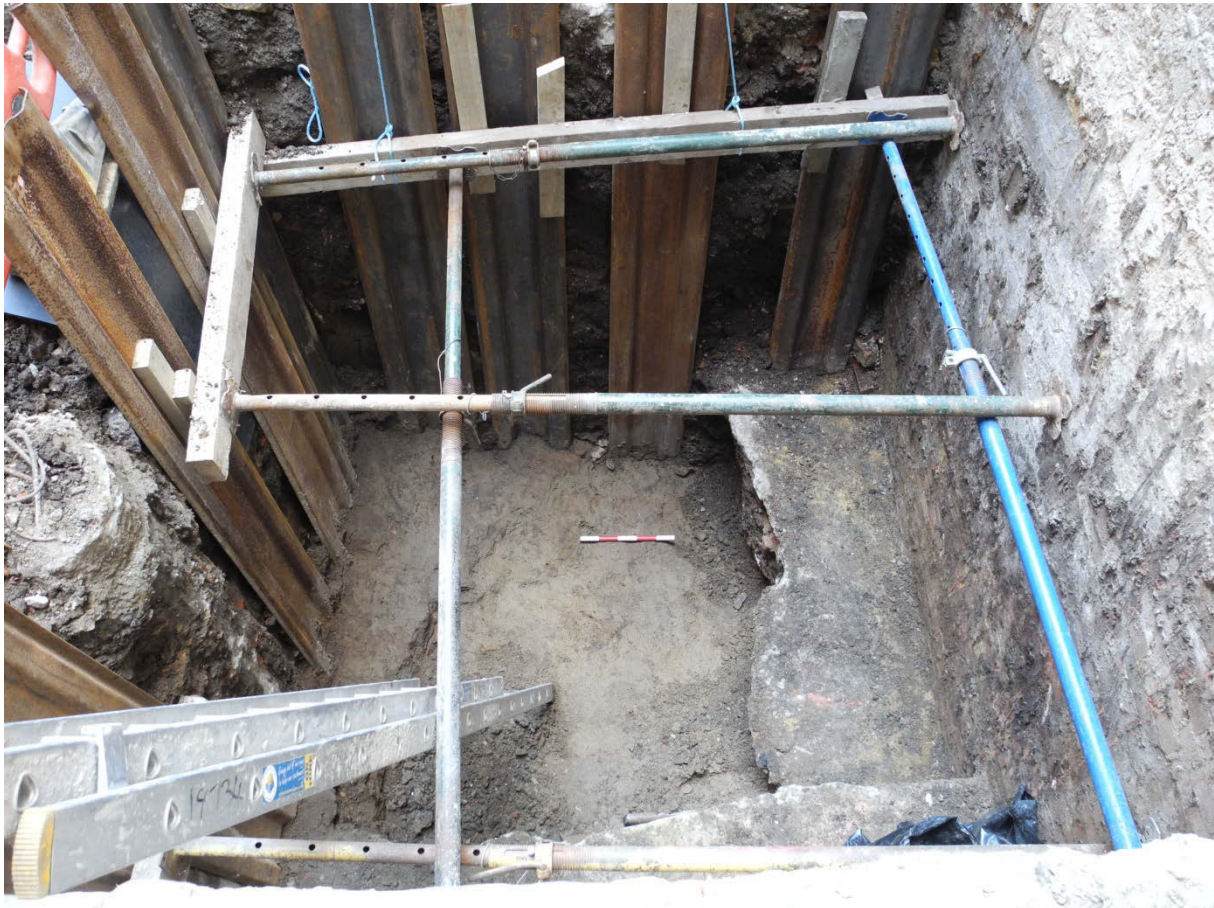
Photo; lift shaft looking west, with scale resting on base of cut [08]
