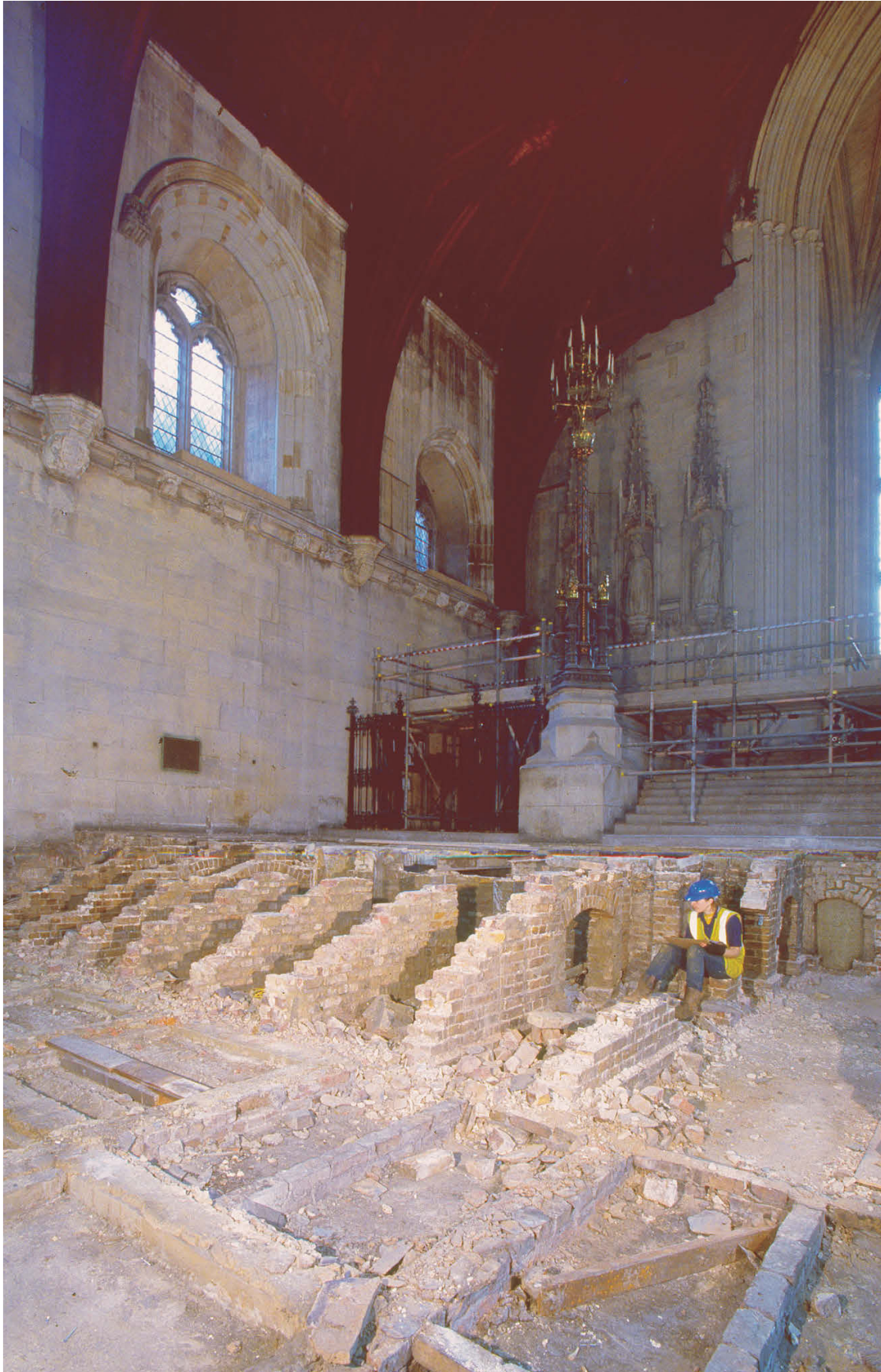
Fig 8 View looking south-east at the 1850s south steps during their dismantling in 2006
